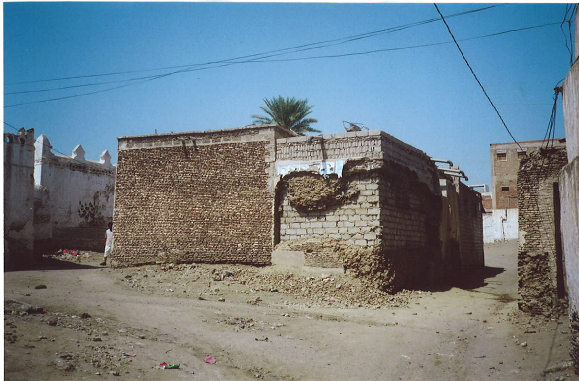
3. Degradation of Canopy on Suq
