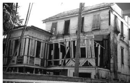
Chess Hall in Georgetown (Guyana): situation in 2002, it collapsed soon after and has disappeared from Georgetown's historic streetscape
