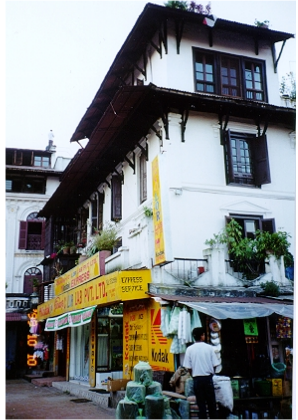
(Above) In October 1998, the original wooden shutters of this building, facing the Patan Darbar Square, were widened and replaced with metal shutters. Simultaneously, the entire ground floor was covered with inappropriate large bright advertisement which is illegal within the protected Monument Zones.
