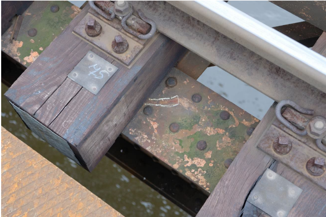
Fig. 11 Fatigue crack in stringer (B. Espion, 11 December 2024 (also in various documents)).
