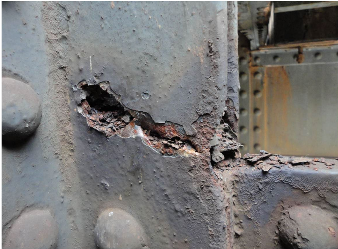
Fig. 12 Example (worst case) of corrosion damage in a vertical (Slide 6 of the presentation by Martin Vlasák from SUDOP PRAHA a.s. on 12 December 2024; similar picture in Slide 25 of the presentation by Ian Firth on 12 December 2024.
