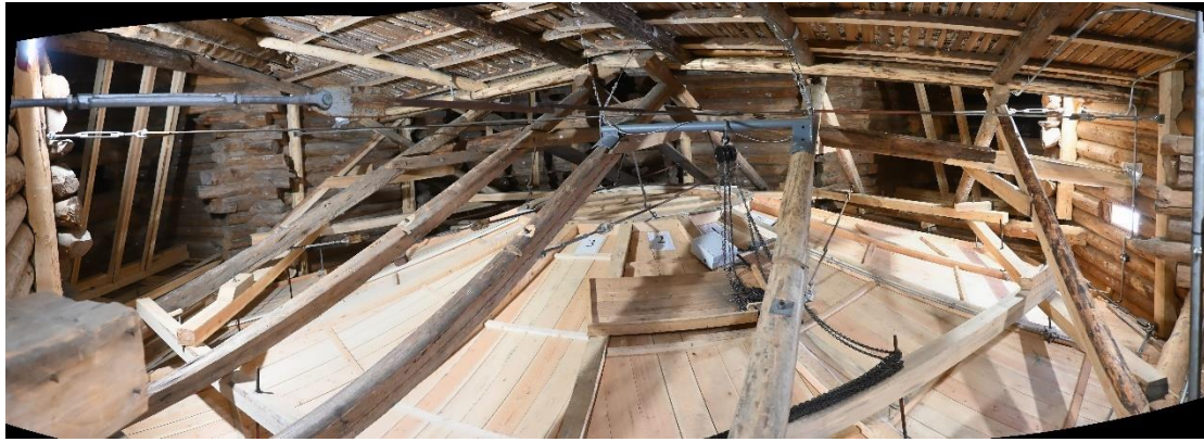
Image 16. View from above the "heaven", with the metallic rod collar and the rainwater evacuation system.
