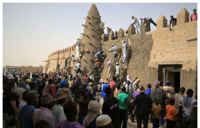
Community-centred approach for the reconstruction of destroyed mausoleums in Timbuktu, Mali. Photo: © UNESCO | Bayoko Modibo
