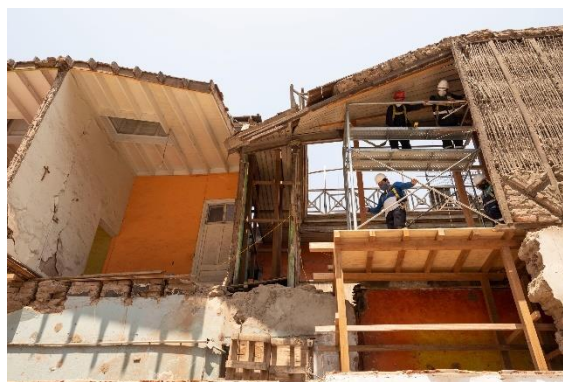
Image 17b: Emergency interventions through Stabilisation work after collapse, fire or imminent danger in HCL buildings
