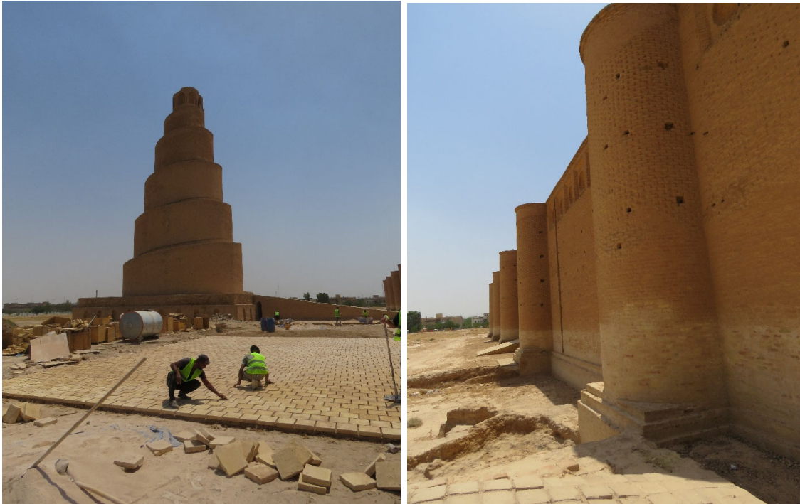
Figures 1 and 2: Views of the ongoing exterior tiling work at the Great Mosque © UNESCO/May Shaer
