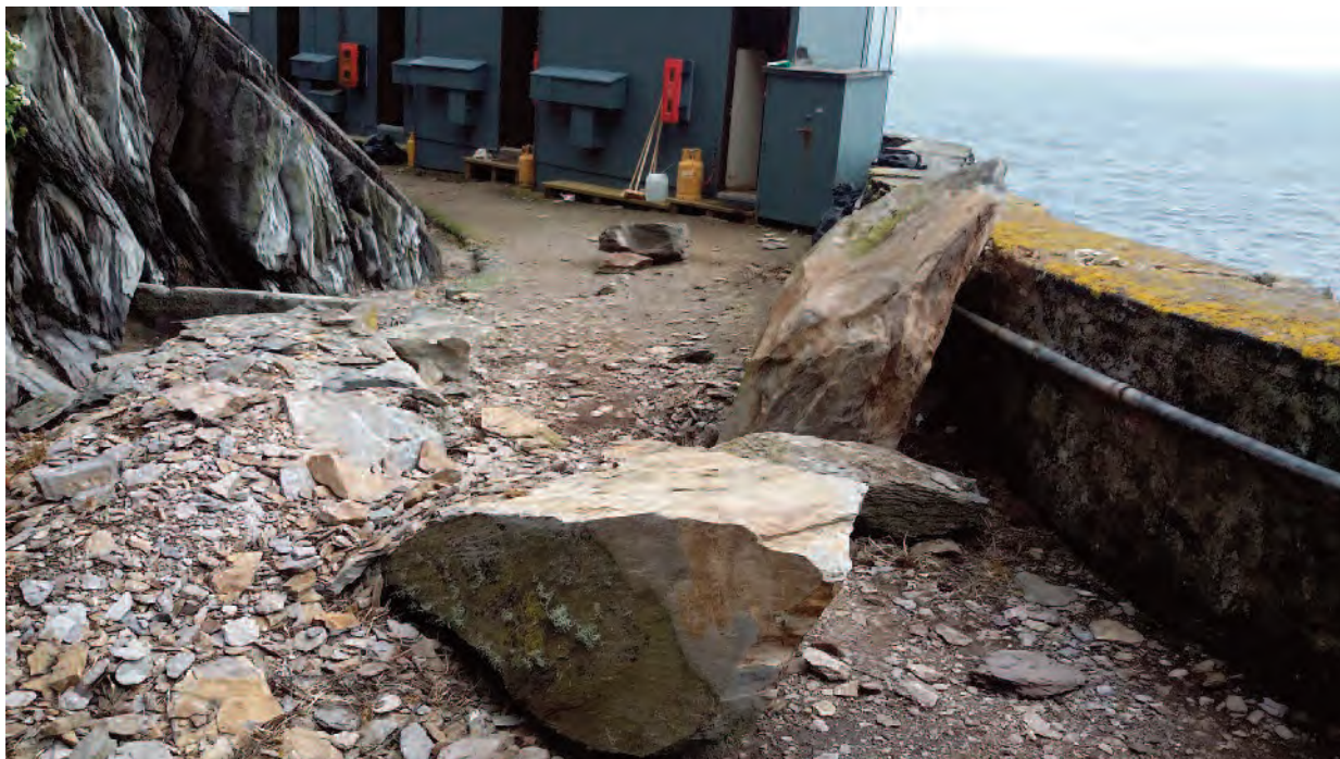
Pl. 26 Rockfall close to staff accommodation.
