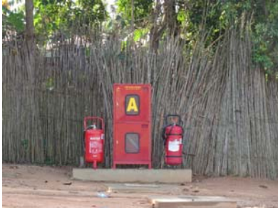
Fire hydrant and extinguishers
