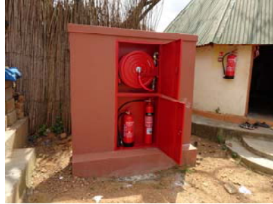
Fire hydrant and extinguishers
