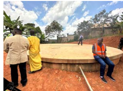
Underground water tank
