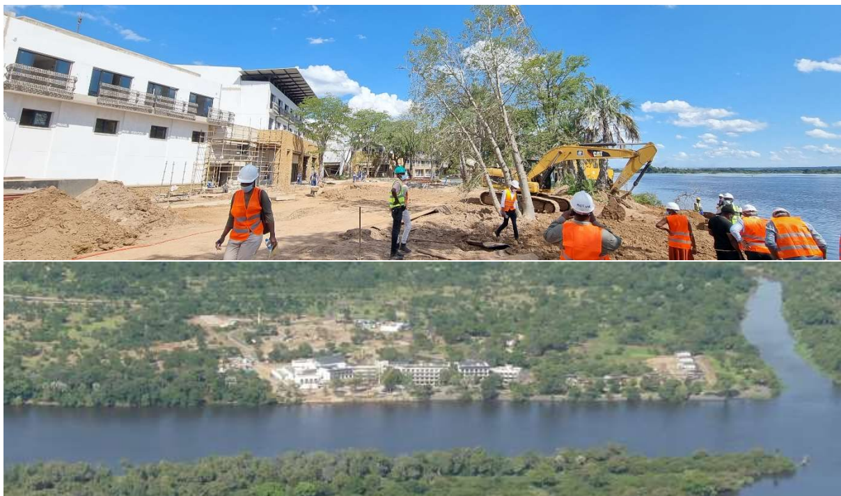
Figure 1. (top) Mosi-oa-Tunya Livingstone resort under construction as of 9 February 2022 adjacent to the Zambezi River; (bottom) aerial view of the resort development taken on 13 February 2022. ©IUCN/Mizuki Murai.
