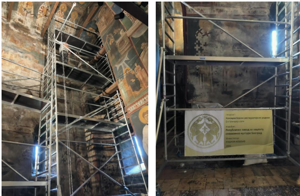
Photos 7 and 8: The organization of the work site, the north wall, and the apse of the proscomidia
