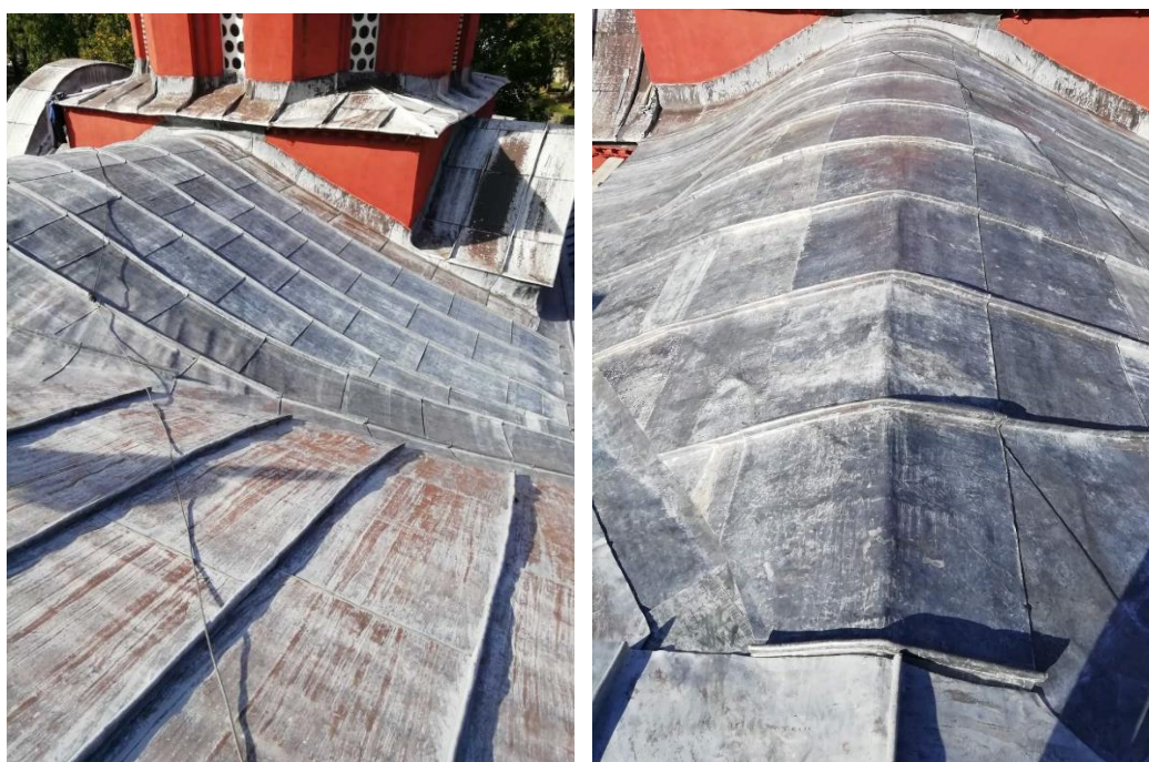
Photos 12 and 13: Roof repairs on the church of St. Apostle in the Patriarchate of Peć Monastery; Photos by Institute for the Protection of Cultural Monuments
