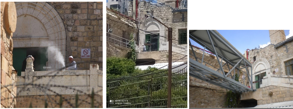
Figure 14: The stone balustrade before and after destruction in order to install the electric elevator
