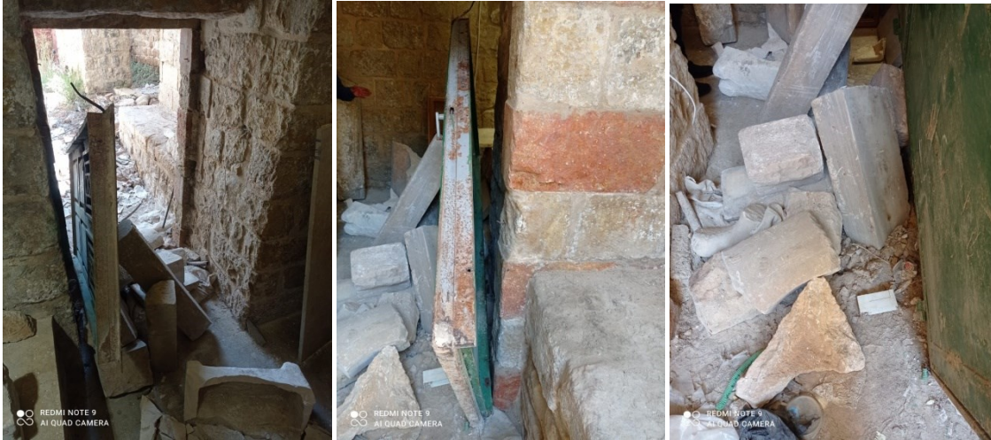
Figure 23: The destruction of the artifacts in the Old Town’s Visitor Center
