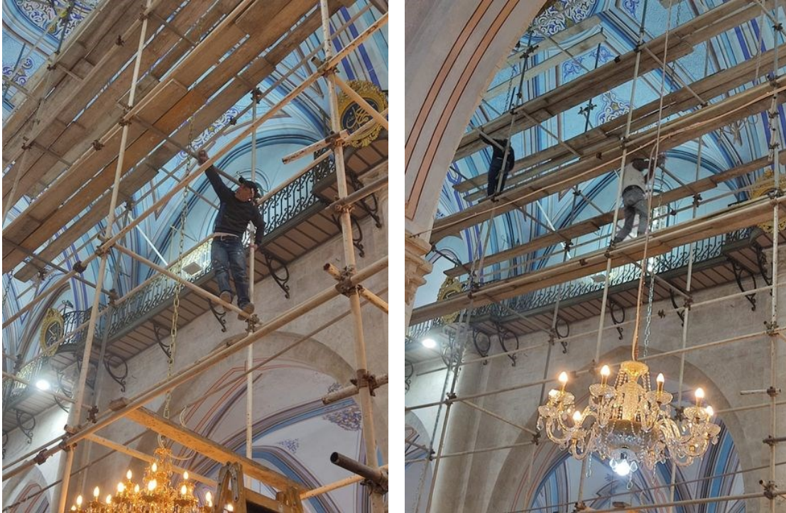
Figure 1: Maintenance of lighting system in the Ibrahimi Mosque/ The Tomb of the Patriarchs
