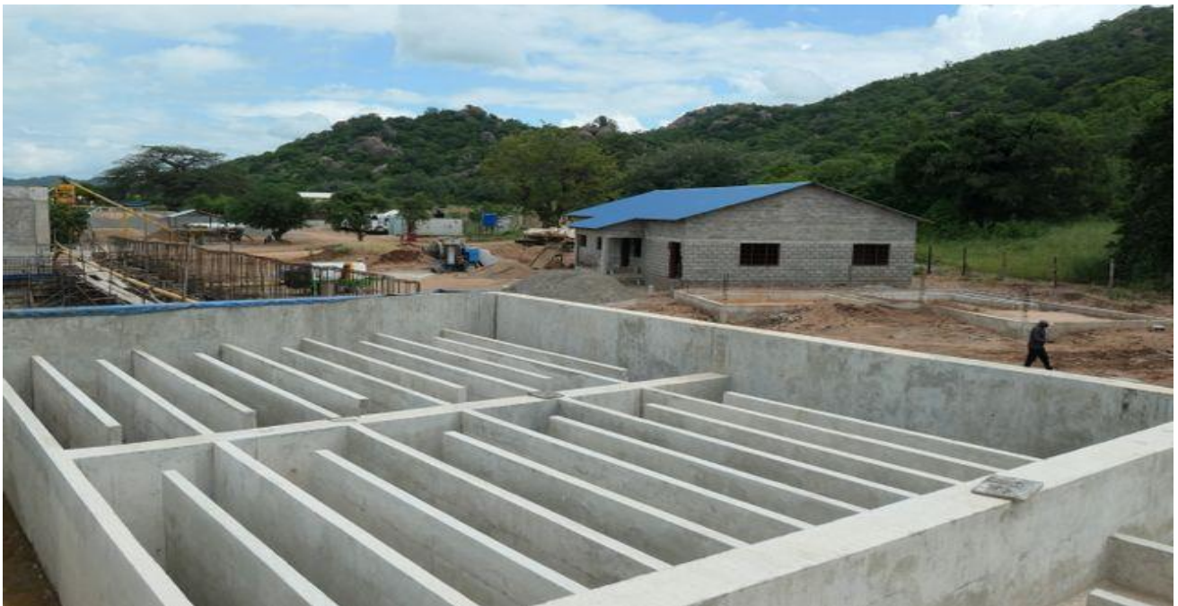
Construction works at the water purification site are at an advanced stage. Photo ©IUCN/Peter Howard
