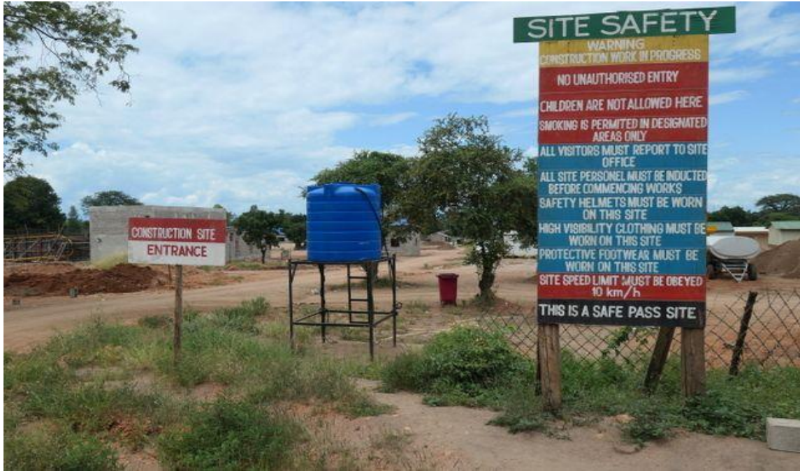
Entrance to the Mangochi Water Supply Scheme water purification construction site, located outside the national park. Photo ©IUCN/Peter Howard
