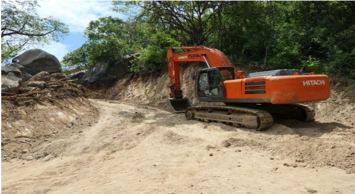
Heavy machinery is still on site to finish the construction works, after which the road will be surfaced carefully in order to blend with the natural environment. Photo ©IUCN/Peter Howard
