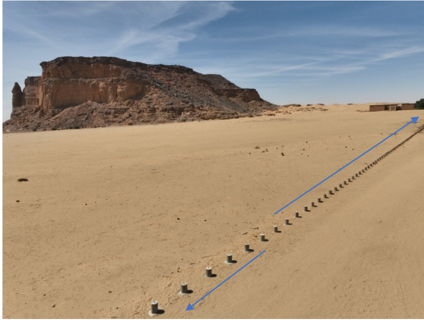
Figure 5: Concrete bollards continue to be installed around the site – 2023 (Drone photo: Sami Elamin)
