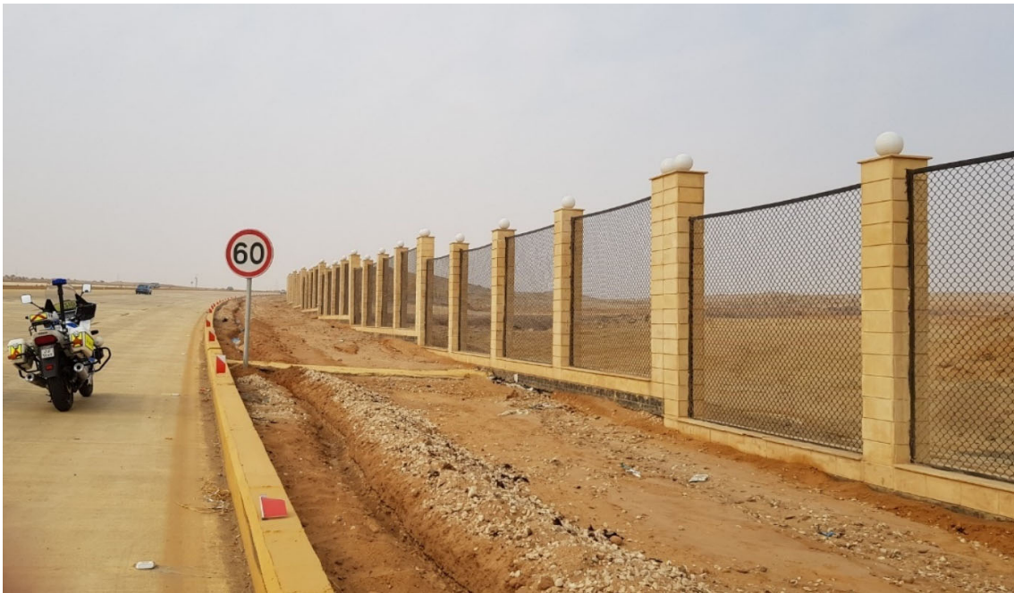
Figure 2: The “Touristic Path” with fence along its northern edge ©ICOMOS / J. Tabet
