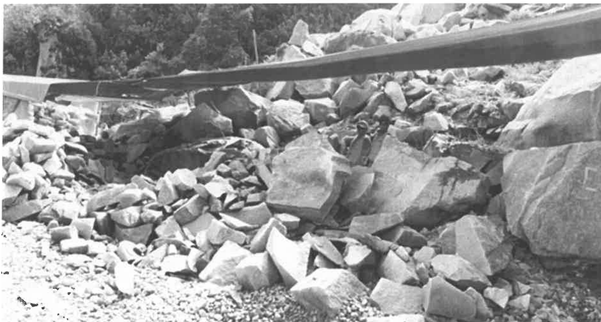
Photo 4.8. Repairs on the side of the Hiram Bingham road after a rockslide
