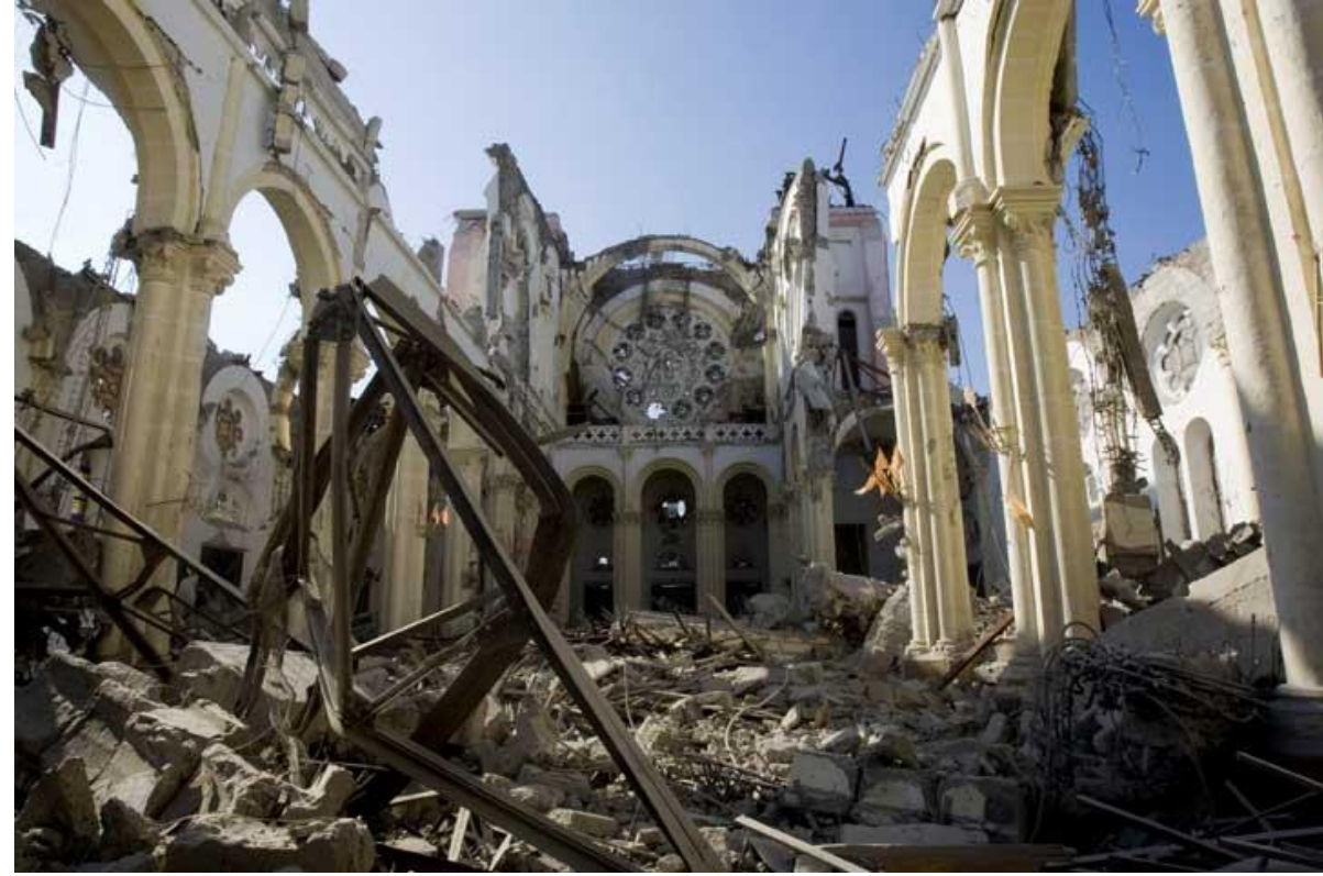
The remnants of the Cathedral of Our Lady of the Assumption in Port-au-Prince (Haiti), destroyed by the 2010 earthquake
