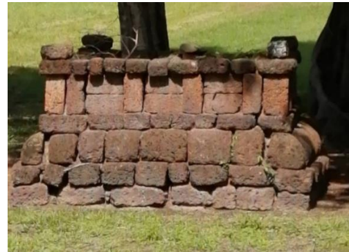
Figure I-3-14 The base of the stone Dharmachakra made of laterite brick laid to form small rooms
