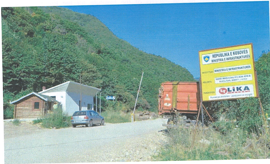
Photo 2: Construction works on the road Dečani – Plav through the Dečani monastery buffer zone, August 2020. Photo by Institute for the Protection of Cultural Monuments
