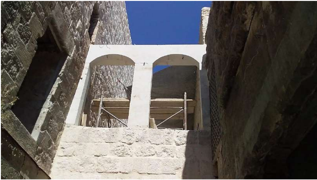
Renovation work on the outer walls of the room above the alley
