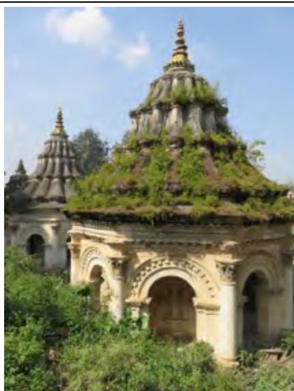
Temples near Bagmati River have not been repaired as yet.
