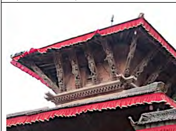
Loose bricks in upper storey of Jagannath Temple
