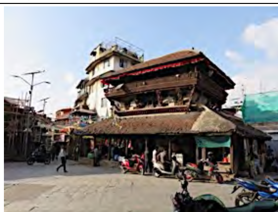
Garud Narayan Temple did not suffer severe damage during the earthquake, but is showing signs of neglect with roof desperately needing repair
