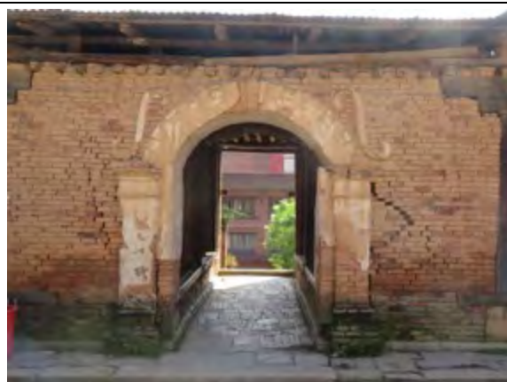
Other side of entrance way through earthquake damaged sattal
