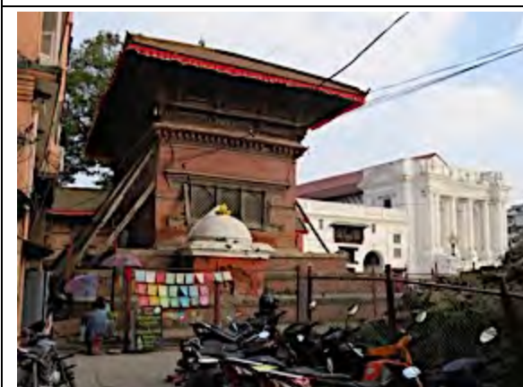
Nava Jogini House is still to be repaired
