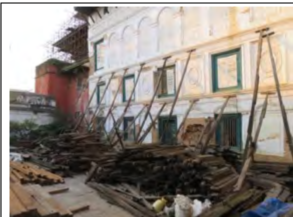
Wing of palace adjoining the Degutale Temple is still in very poor condition and yet to be fully stabilised and repaired
