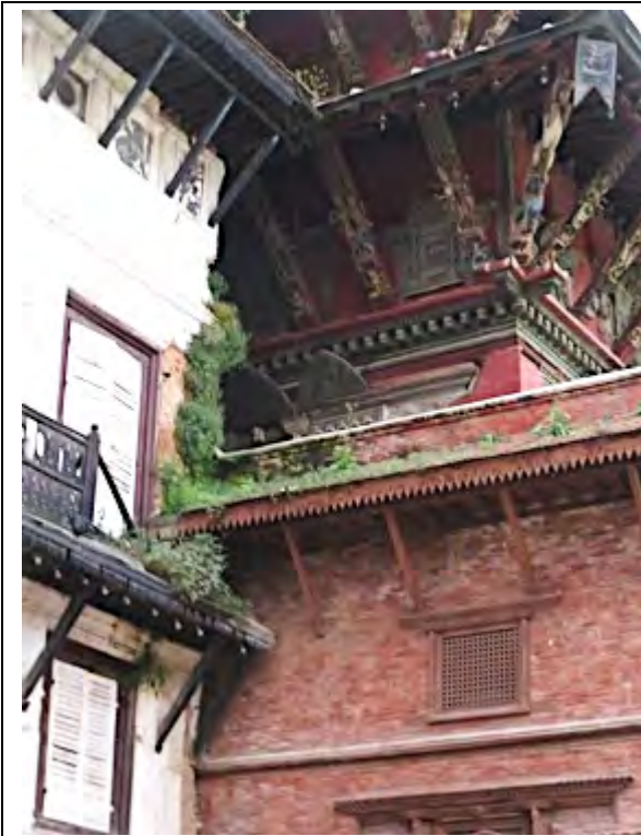
Falling damp affecting palace and Degutale Temple as palace wing has not been repaired as yet
