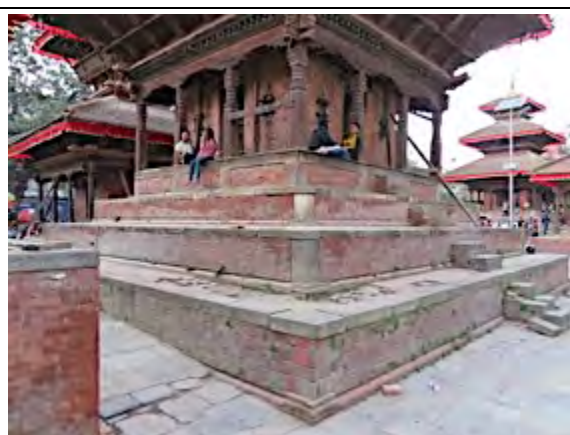
Temporary stabilisation and safety barriers removed from Shree Krishna Mahavishnu Temple, which has damage to its lower structure
