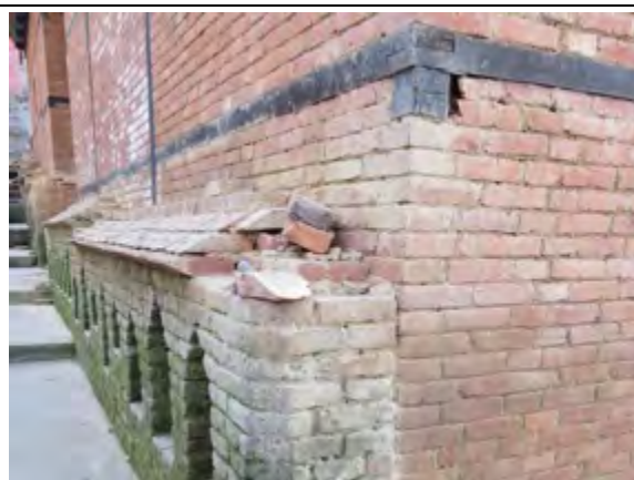
Monkeys lift plinth bricks laid in mud mortar, making it difficult to maintain the brickwork of the temple.
