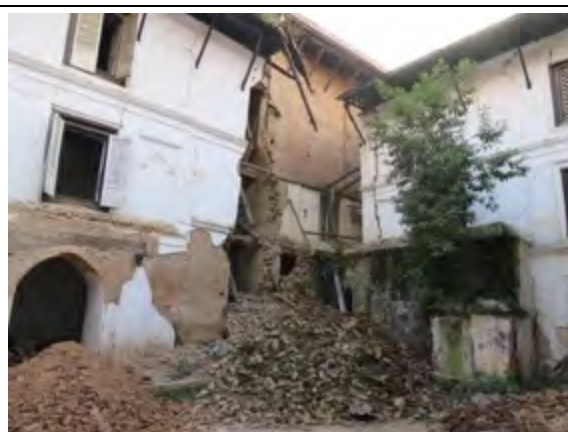
Section of palace that has collapsed since the 2017 RMM due to exposure of walls to the weather
