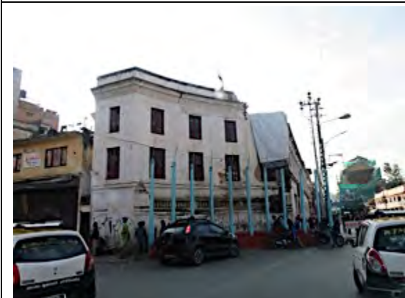
East elevation of the fire station showing partial collapse due to the earthquake and prolonged exposure to the weather. This building is within the Monument Zone.
