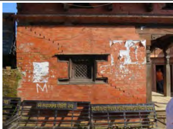
Earthquake damage to rest house
