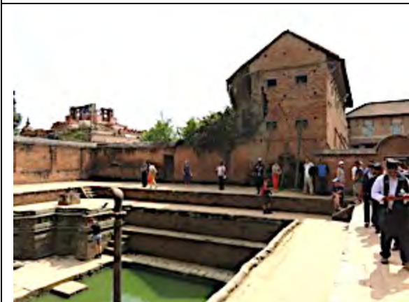
Municipality building (right) has suffered partial collapse since the 2017 mission due to exposure to the weather. The hitti has been restored.
