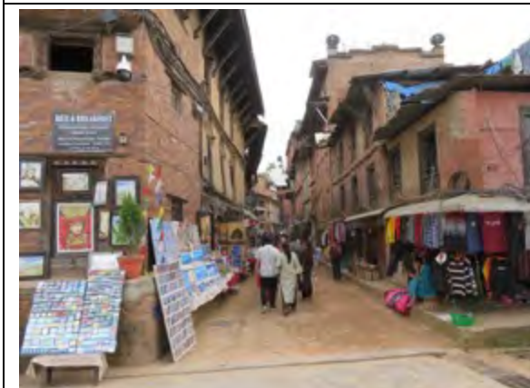
Earthquake damaged traditional houses near Dattatreya Square remain unrepaired (right)
