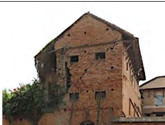
Damage to Municipality building located to the rear of the Fifty-five Window Palace
