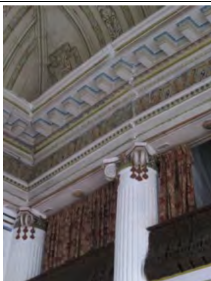
Structure of Gaddi Baithak has been stabilised. Crack and dislocation in eastern end wall has been left as evidence of the earthquake.
