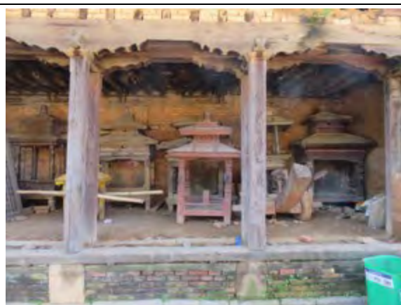
Movable heritage items stored in dilapidated sattal on eastern side of temple courtyard
