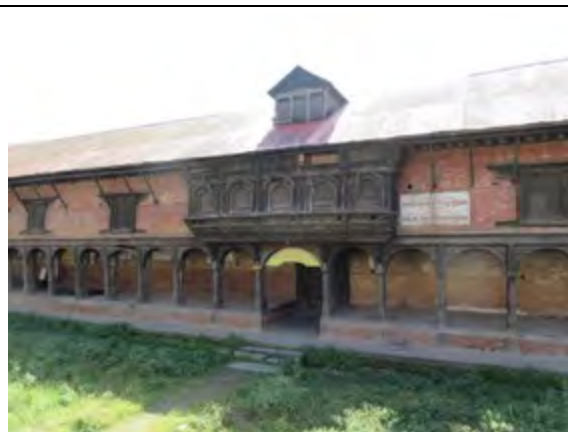
This building has been vacated to allow repairs to be carried out.
