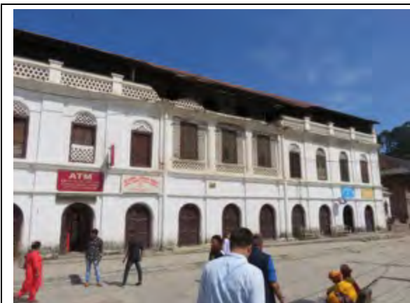
Damage to this early twentieth century building, located adjacent to the main path down to the river, has not been repaired as yet.
