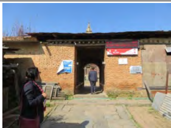
Eastern entrance to temple complex – brickwork has been repaired, but is missing its original detail; upper floor of sattal is still missing; new electronic signage has been mounted on the wall adjacent to the entrance and is intrusive to the temple context
