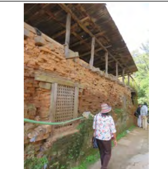
Rear wall of northern sattal has lost its external skin of brickwork
