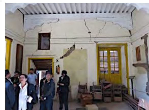
Damage to Lal Baithak is being monitored, but repairs have not been undertaken.
