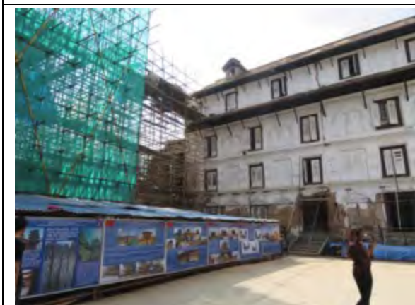
Southern wing of palace (left, scaffolded) has been substantially demolished as a result of the earthquake damage and decay resulting from ongoing exposure to the weather – to be rebuilt.
