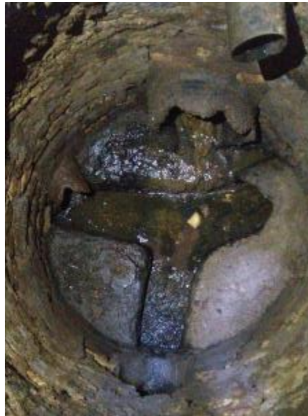
Figure 9. Destruction and decay of the sewage pipe in the area of the Emam square, point 1 in Figure 1
