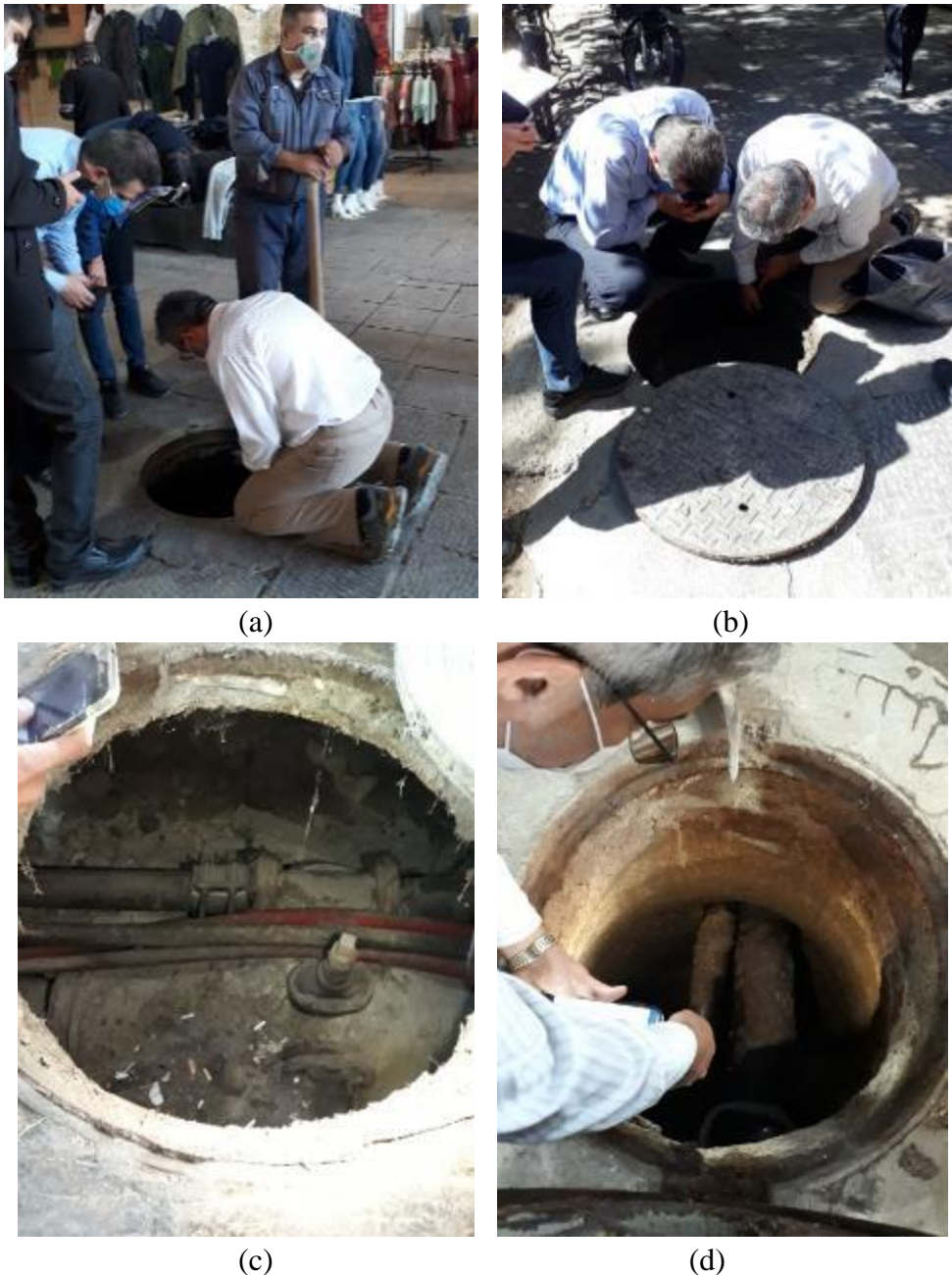
Figure 7. Investigation of manholes in the area of the Emam square, point: a) 5, b) 7, c) 4, d) 6 in Figure 1
