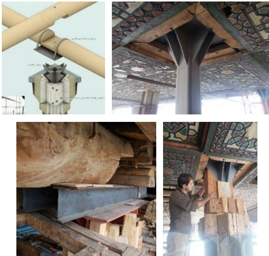
Figure 21. Ali Qapu edifice, strengthening the connections of the columns to top beams (2005 to 2017)
