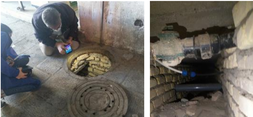
Figure 6. Water pipeline crossing the area of the Emam square, point 2 in Figure 1
