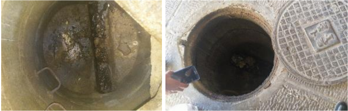
Figure 11. Existence of plastic containers in the sewage path and the low slope of the sewage pipeline, point 9 in Figure 1
