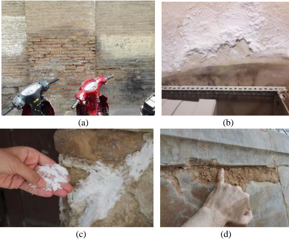
Figure 10. Leakage effects from sewage pipes, point a) 9, b) 10, c) 3, d) 11 in Figure 1
