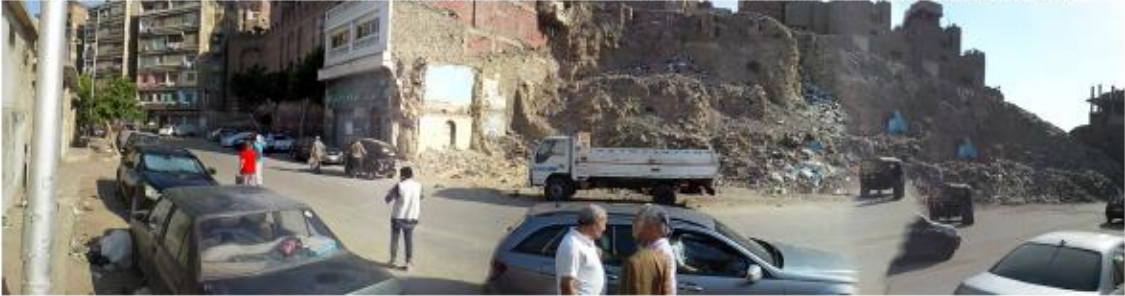
1 Extensive demolitions in Abd al-Maguib el-Labban have defigured the layout of the street
