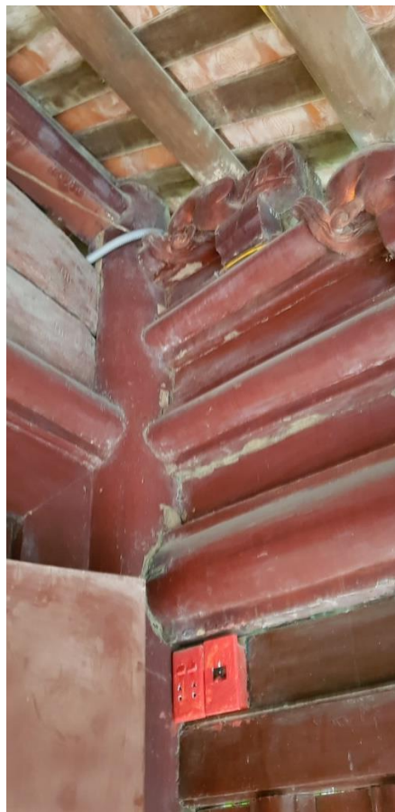
© Andrew Sneddon, 2019 – Intrusive wiring and electrical hardware (possibly a fire risk) at the Hoa Lu Ancient Capital temples
