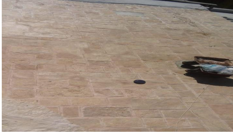
Maintenance & Cleaning works for the roof of Al- Haram Al-Ibrahimi/Tomb of patriarchs
