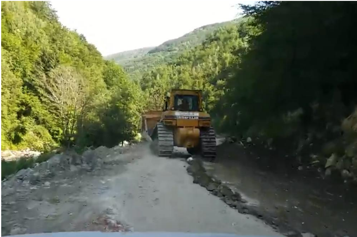
1. Construction works on the road Decani – Plav through the Dečani monastery buffer zone, May 2018
