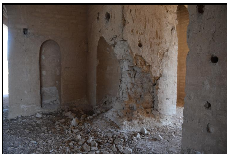
Figure 8: Effects of damages in Qubbat al-Sulaibiyya as a result of the 2014 clashes.
