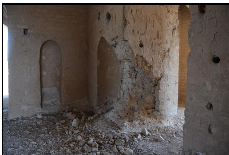
Figure 8: Effects of damages in Qubbat al-Sulaibiyya as a result of the 2014 clashes.
