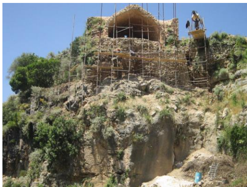
The damaged tower before restoration
