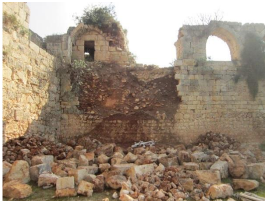
The collapsed part of the byzantine wall on the southeastern side of the castle - before
