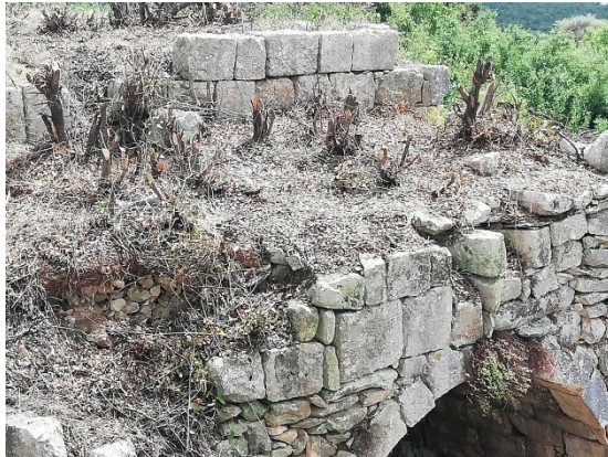
Structural problems such as cracks, stone and mortar loss
