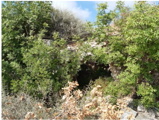
The trees density cause cracks in the structure
