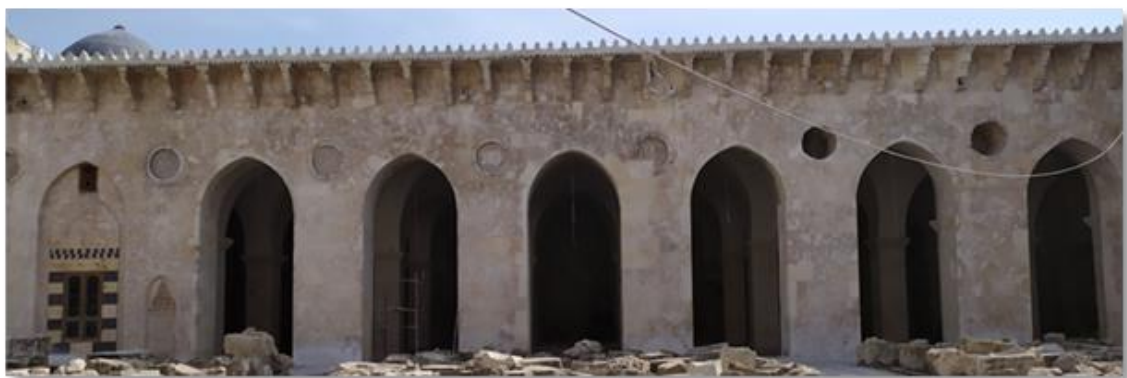
The restoration of the Eastern Rewaq façade by cleaning the holes from metal shrapnel and filled with traditional mortar, then filling with lime mortar and hammering a stone of the façade.
