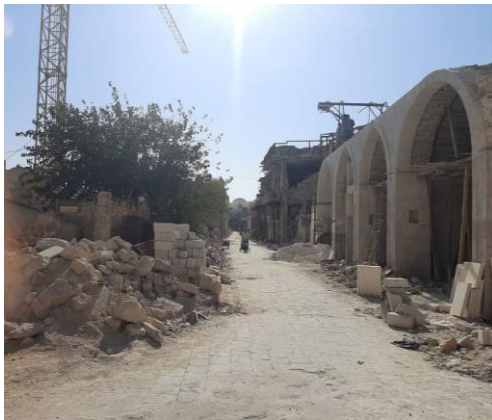
The damage at the Al-Haddadeen Souk
