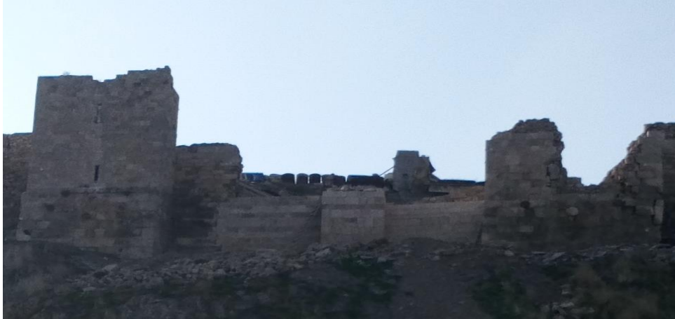
The damaged eastern defenses wall of the citadel of Aleppo before and during the restoration works
