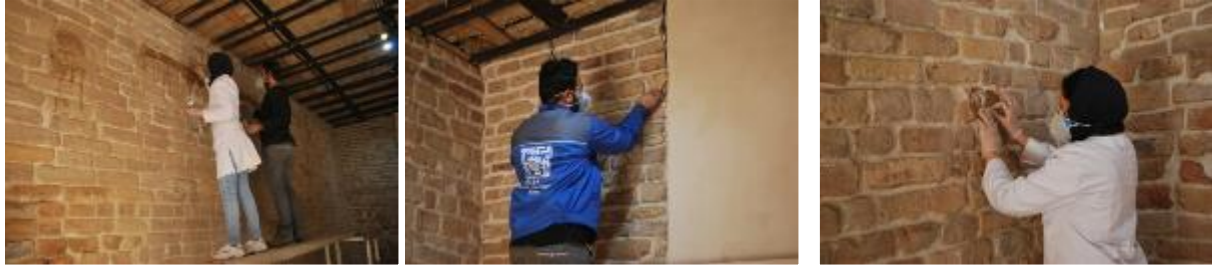
Figure 68. Steps of cleaning and stabilization of brick inscriptions in the Girshman Garage
