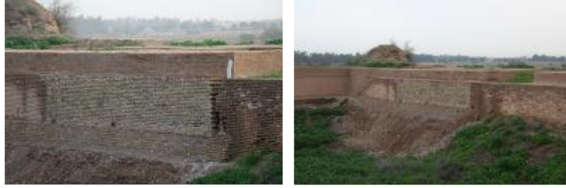
Figure 40 . Local restoration and reinforcing walls of trenches made in yards of Apadana Palace- After restoration
