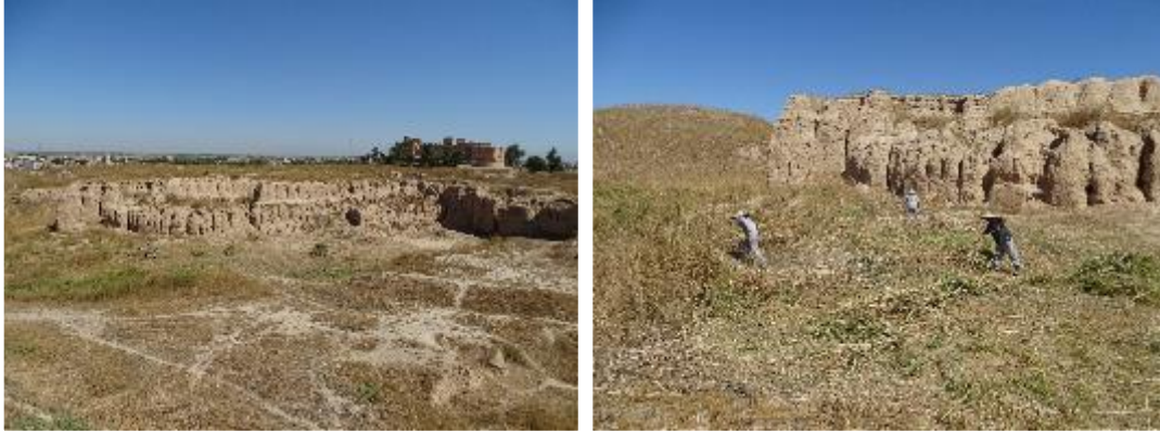
Figure 38. Removing dried vegetation around the mud-laid platform known as high platform of Acropolis hill
