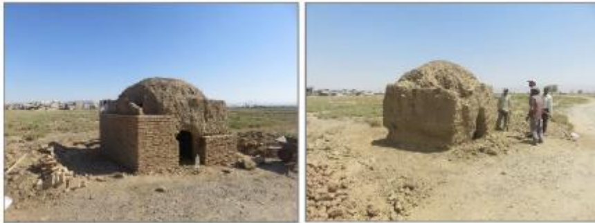
Figure 34. Cutting worn out sections of Baladeh shelters in urban area (right) and reinforcing walls and surrounding wall with mud bricks (left, 2019).
