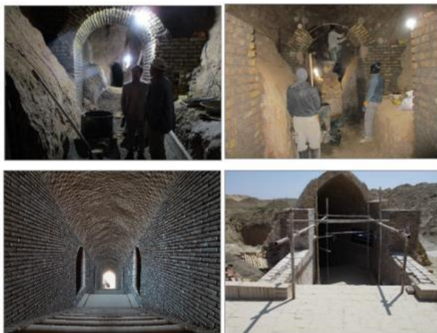
Figure 20. Development of phases 2 and 3 for reinforcing inflowing gate no.2 of Qasabeh Qanat (2018-2019)
