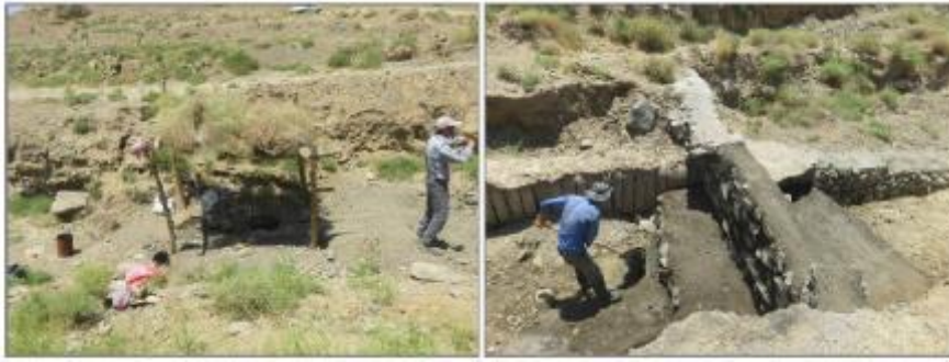
Figure 29. Constructing water dike to control flood flow rate in vicinity of Qanat path (right) and dredging well share and Zane Qanat Gallery (left, 2018)
