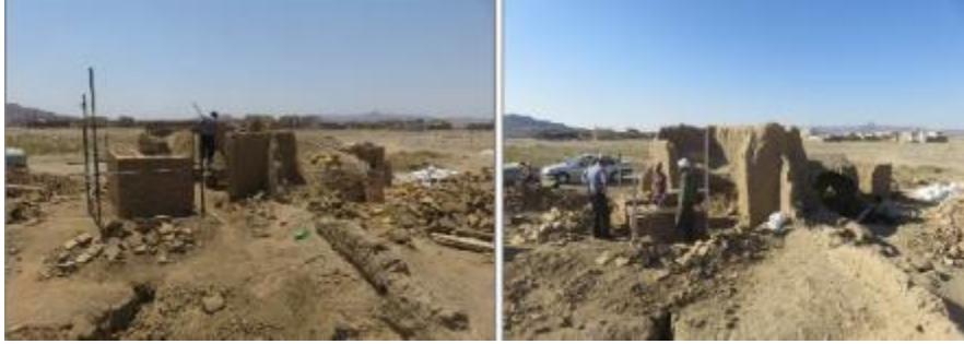
Figure 33. Restoration of Mardkhane and water storage from available materials in Baladeh (right) and construction of destroyed pool roof and laying bricks walls for it (left, 2019)
