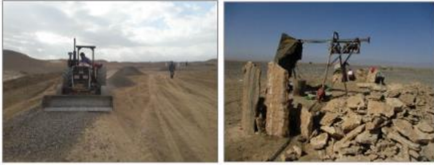
Figure 21. Reinforcing and dredging of Qasabeh Qanat (right), dropping sand and flattening of main touristic route (left, 2018)
