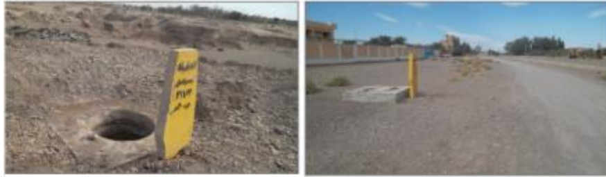
Figure 43. Manufacturing and installation of opening lid for a number of well shafts (2018)
