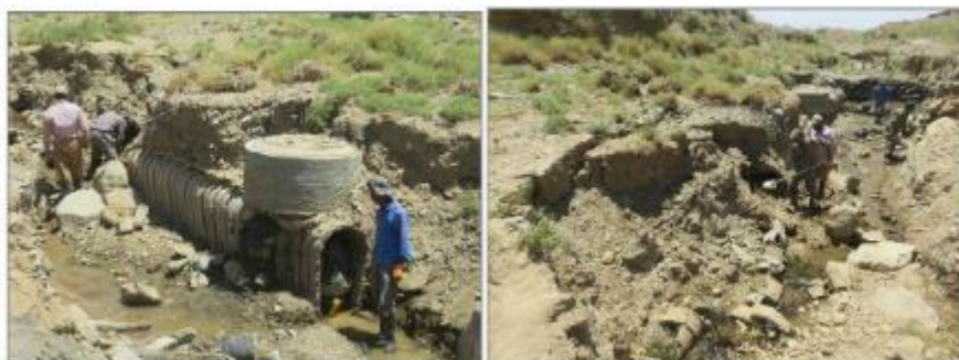
Figure 28. Removing collected debris inside of coils of Zaneh spring coil (right) and substitution of broken coils and restoring them (right, 2018)
