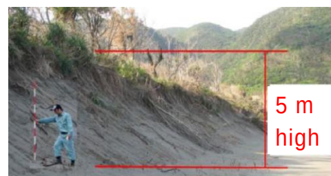
Erosion caused by typhoons
