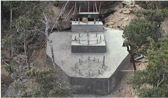
Figure 9: trees still growing right next to the footings during construction
