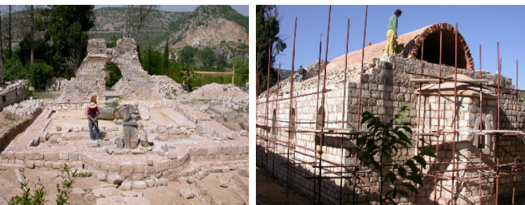
Figures 16 (left) and 17 (right). Reconstruction process at the site and remains of the sixteenth century Eastern Orthodox Monastery in Žitomislíci. © Commission to Preserve National Monuments of Bosnia and Herzegovina
