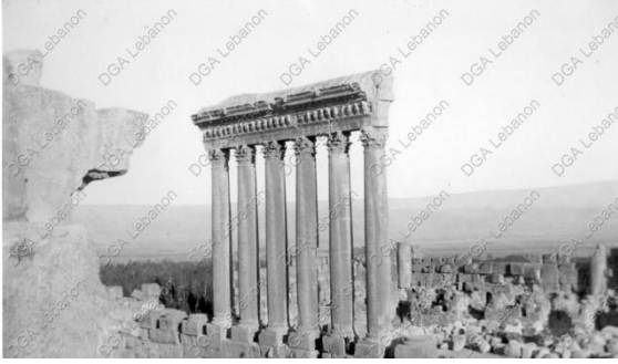
Figure 20 – View of the newly consolidated Jupiter Colonnade after the scaffolding has been removed as shown from the southeast. The concrete cap with its thickened portion and the westernmost span can be seen as well as the building up of the stone lintel on the east (right) to further consolidate the bearing of the stone lintel on the easternmost column. Photograph taken during the French Mission, circa 1930s.
