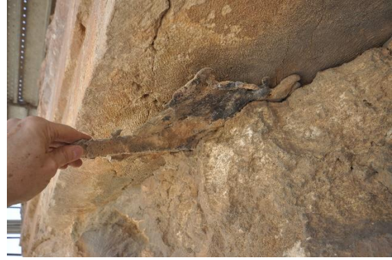
Figure 27 – Some of the molten lead within the stone lintel (between architrave and freeze stone units). Has been exposed on the north side.
