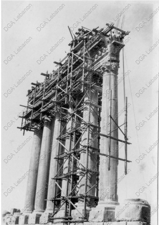
Figure 11 – View of the Jupiter Colonnade as seen from the southeast with wooden scaffolding in place. A suspended wooden scaffolding hangs from the top of the stone lintel to facilitate work on the architrave and frieze. Photograph taken during the French Mission, circa 1930s.
