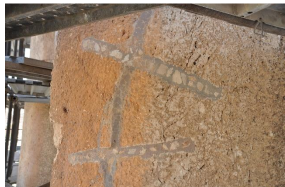
Figure 29 – Area where staple shaped metallic anchors were embedded spanning a vertical crack in one of the capitals.
