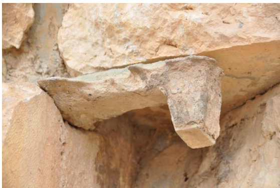
Figure 35 – Roman era cast bronze anchor set in lead that has been exposed due to previous damage on the north side of the stone lintel in the horizontal joint between the architrave and frieze stones.
