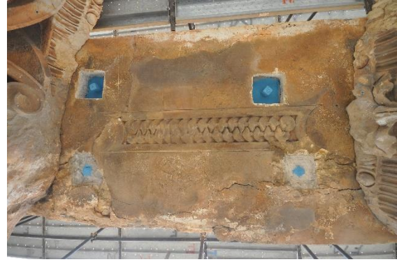
Figure 41 – View of the underside of another one of the architrave stones that has been suspended from the reinforced concrete cap above.
