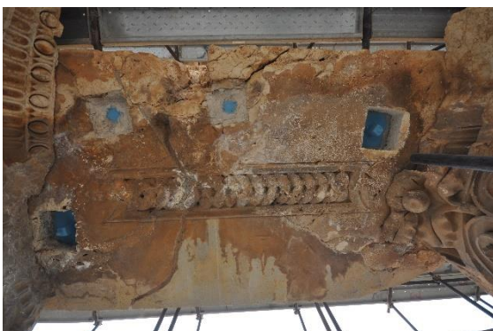
Figure 40 – View of the underside of the westernmost architrave stone which had been compromised by a large crack.
