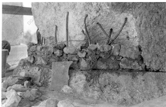
Figure 12 – Work in progress at the base of one of the damaged columns. Ferrous metal rods have been set in drilled holes in the column stone, and the exterior face is filled with limestone laden mortar. The cavity behind the face is believed to be filled with concrete. Photograph taken during the French Mission, circa 1930s.
