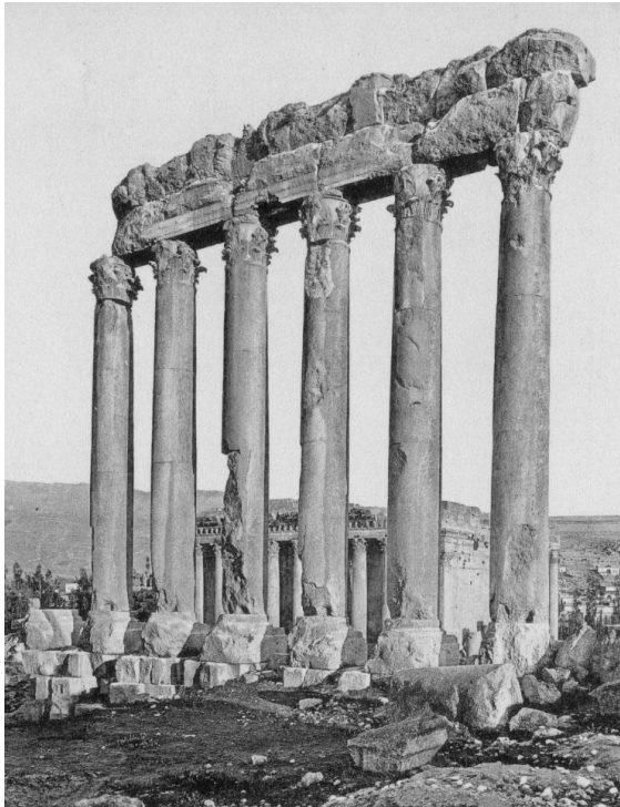
Figure 8 – View of the Jupiter Colonnade as seen from the north. The unconsolidated stone lintel reveals the extensive amount of stone loss and the tenuous nature of the stone lintel bearing on the easternmost column (left). In addition extensive damage can be seen emanating from the base of several of the columns which is most likely resultant from the rocking of these columns during seismic actions. Photograph taken during the German mission, circa 1900.
