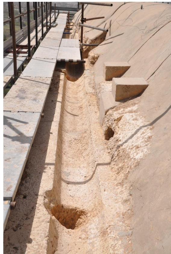
Figure 42 – The original guttering system within the stone frieze. The concrete cap allows water to drain into this guttering system which has downspouts that lead to the mouths of carved lions in the south side of the frieze.
