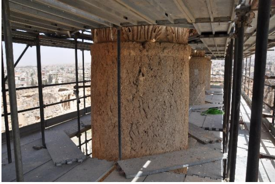
Figure 25 – Alveolarization of the limestone on the face of the column shaft just below the capital.
