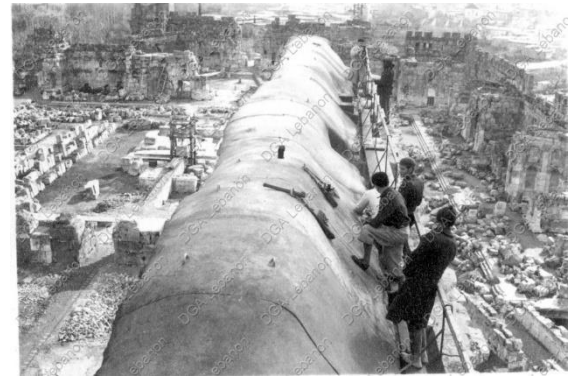
Figure 19 – View of the reinforced concrete after it has been poured as seen from the west. Control joints in the concrete cap mimic the joints between the stones of the frieze upon which it has been cast. The concrete cap was finished by hand without formwork so that it would shed water. Metallic anchors protrude from the top to assist in access and repair work that may be planned in the future. Photograph taken during the French Mission, circa 1930s.
