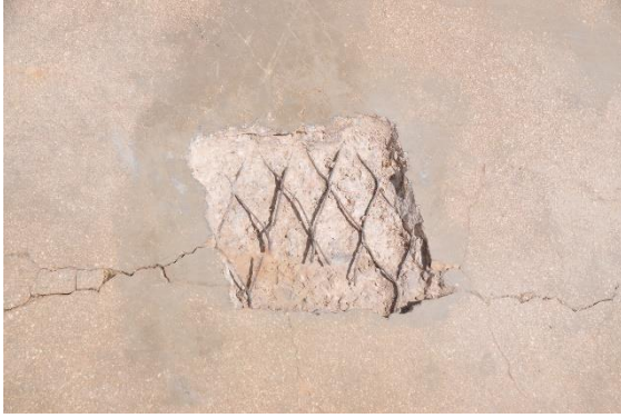
Figure 43 – Welded wire fabric was placed in the concrete cap near the surface to control shrinkage cracks in the concrete and increase its water shedding abilities.
