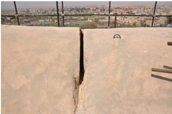
Figure 44 – Formed break in the concrete cap towards the west end of the cap. Little is known about the steel reinforcing within the concrete other than it must be present above the architrave stones that are suspended and is discontinuous at this break.
