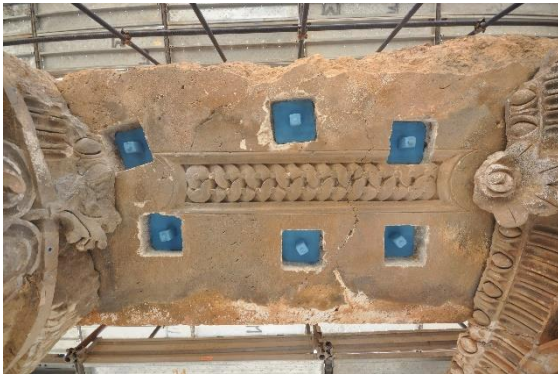
Figure 39 – View of the underside of one of the architrave stones that has been suspended from the reinforced concrete cap above. Through plates, recently painted blue, were inset into the stone and then covered with mortar.
