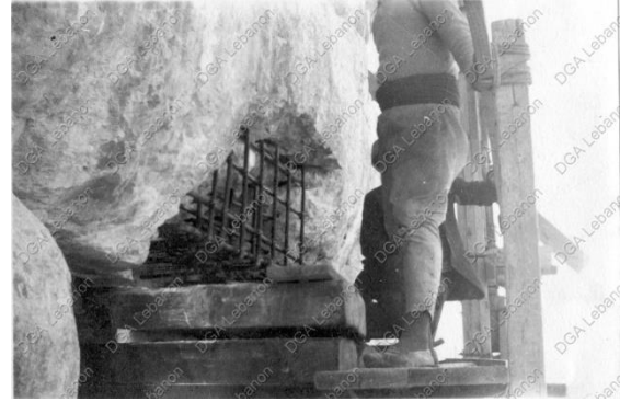
Figure 13 – View of the underside of the stone lintel on the north side where extent extensive stone loss is being replaced with reinforced concrete. Photograph taken during the French Mission, circa 1930s.
