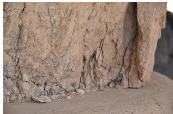
Figure 28 – Close up view of the north side of one of the column shafts where it rests on the base. This is an area where the stones have been damaged possibly due to rocking during seismic actions. It appears that this damage may be exacerbated by freeze thaw decay.
