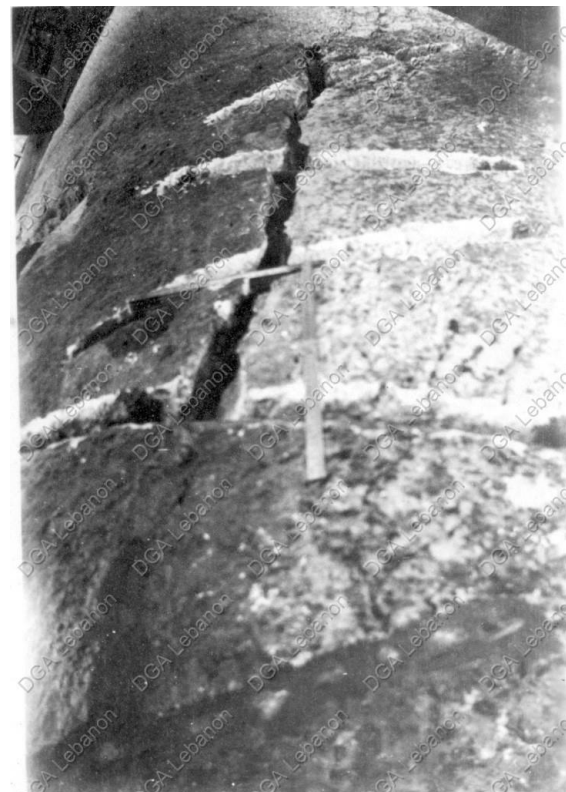
Figure 14 – Staple shaped ferrous anchors embedded in slots that span a vertical crack on the south side of one of the columns. Photograph taken during the French Mission, circa 1930s.
