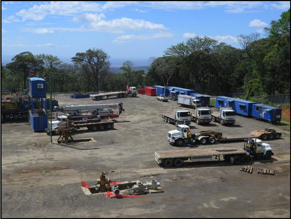
Photograph 5: Las Pailas II geothermal project by ICE on the boundary of Rincón de la Vieja National Park. ©IUCN/Tilman Jaeger
