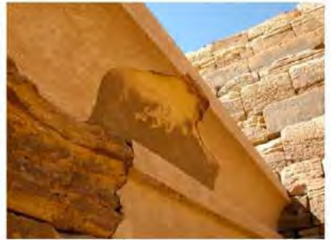
DSCN3752.JPG, Failure of Past Repair Work, Northern Cemetery
