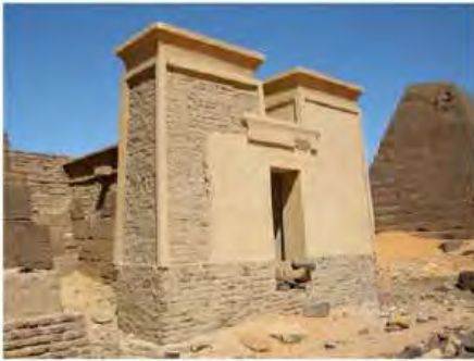
DSCN3798.JPG, Failure of Past Repair Work, Southern Cemetery
