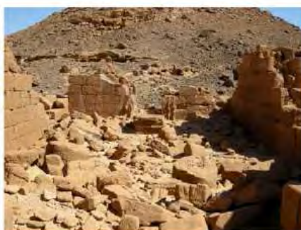
DSCN4147.JPG, Naqaa, Temple F, Structural Instability of Walls/Collapse of Archaeological Features, Structural Instability of Walls/Collapse of Archaeological Features
