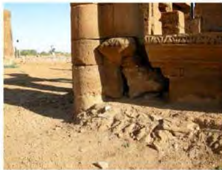
DSCN4003.JPG, The Kiosk - Naqaa, Naqaa, Degradation of Stone/ Masonry Elements, Inappropriate/Inexistent Site Drainage
