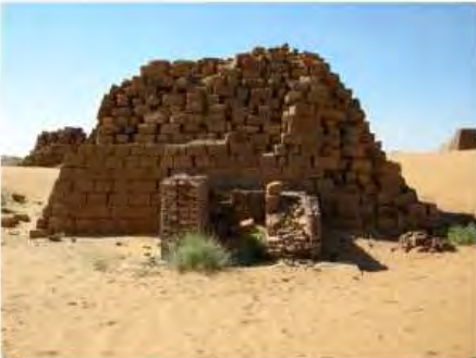
DSCN3836.JPG, Structural Deterioration of Pyramids, Failure of Past Repair Work, Southern Cemetery
