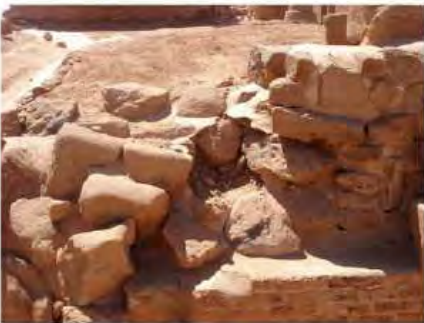
DSC06198.JPG, Musawwarat - Great Enclosure, Restoration Works, Structural Instability of Walls/Collapse of Archaeological Features
