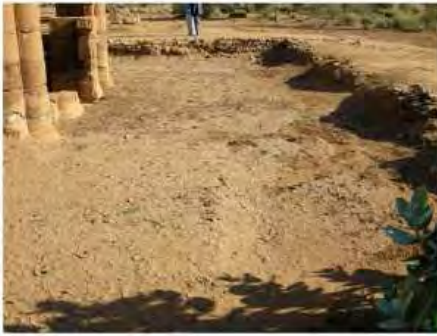
DSCN3999.JPG, The Kiosk - Naqaa, Naqaa, Degradation of Stone/ Masonry Elements, Inappropriate/Inexistent Site Drainage
