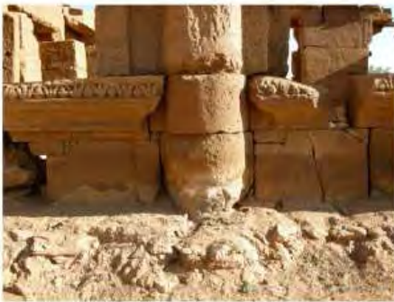
DSCN4002.JPG, The Kiosk - Naqaa, Naqaa, Degradation of Stone/ Masonry Elements, Inappropriate/Inexistent Site Drainage
