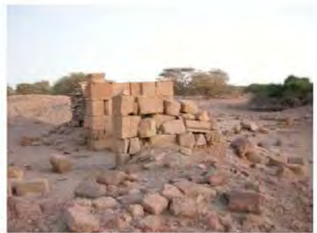
DSCN3988.JPG, Structural Instability of Walls/Collapse of Archaeological Features, Royal City
