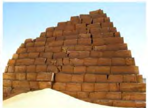
DSCN3740.JPG, Structural Deterioration of Pyramids, Northern Cemetery
