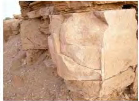
DSCN3958.JPG, Degradation of Stone/Masonry Elements, Structural Instability of Walls/Collapse of Archaeological Features, Royal City
