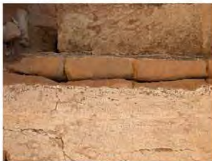
DSCN4153.JPG, Naqaa, Temple F, Exposure and Deterioration of Ancient Plasters, Water Damage
