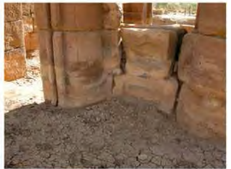
DSCN4004.JPG, The Kiosk - Naqaa, Naqaa, Degradation of Stone/ Masonry Elements, Inappropriate/Inexistent Site Drainage
