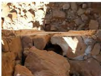
DSCN4156.JPG, Naqaa, Temple F, Structural Instability of Walls/Collapse of Archaeological Features, Structural Instability of Walls/Collapse of Archaeological Features
