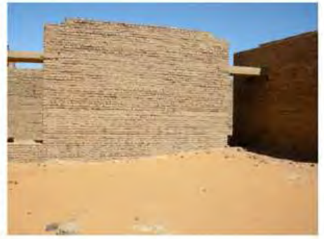
DSCN3818.JPG, Redundant/Inappropriate Visitor Infrastructure
