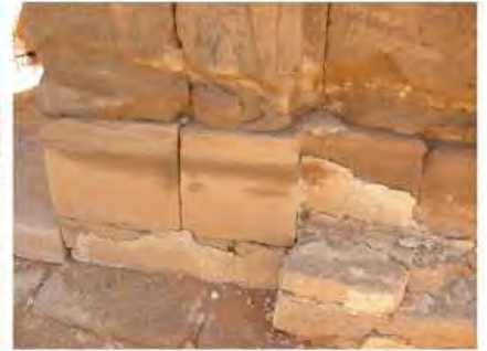
DSCN4092.JPG, Naqaa, Amun Temple, Exposure and Deterioration of Ancient Plasters, Degradation of Stone/Masonry Elements
