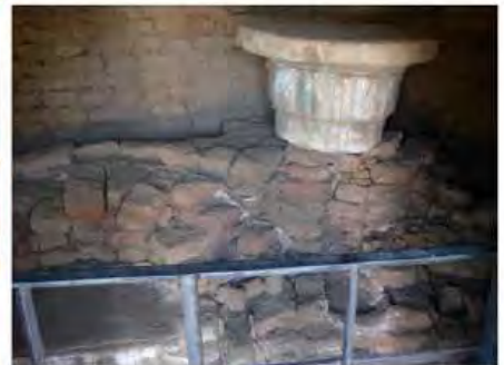
DSC06267.JPG, Degradation of Stone/Masonry Elements, Exposure and Deterioration of Ancient Plasters, Royal City
