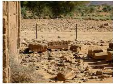
DSCN4043.JPG, The Kiosk - Naqaa, Naqaa, Inappropriate/ Inexistent Site Drainage, Degradation of Stone/Masonry Elements
