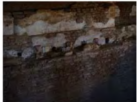
DSC06254.JPG, Exposure and Deterioration of Ancient Plasters, Degradation of Stone/Masonry Elements, Inappropriate/Inexistent Site Drainage, Royal City
