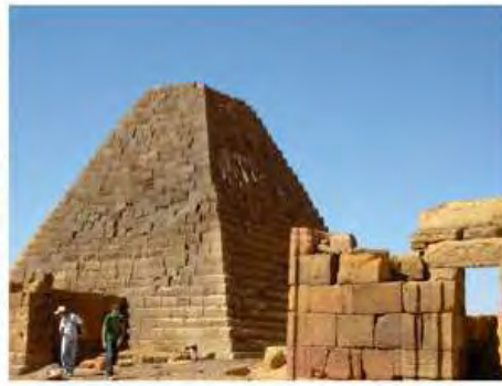
DSCN3769.JPG, Structural Deterioration of Pyramids, Northern Cemetery
