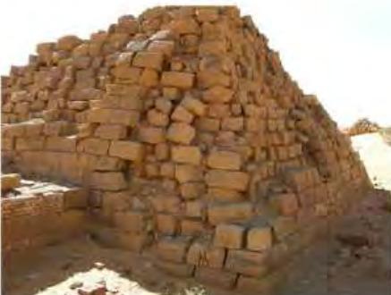
DSCN3839.JPG, Structural Deterioration of Pyramids, Southern Cemetery
