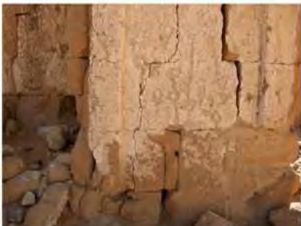
DSCN4151.JPG, Naqaa, Temple F, Exposure and Deterioration of Ancient Plasters, Structural Instability of Walls/Collapse of Archaeological Features, Structural Instability of Walls/Collapse of Archaeological Features
