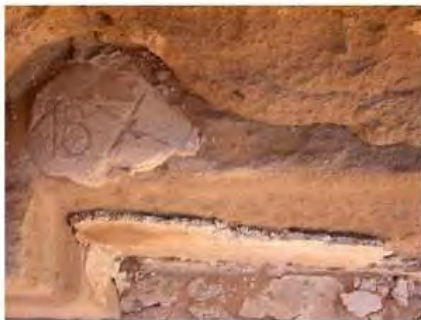
DSCN4093.JPG, Naqaa, Amun Temple, Exposure and Deterioration of Ancient Plasters, Degradation of Stone/Masonry Elements
