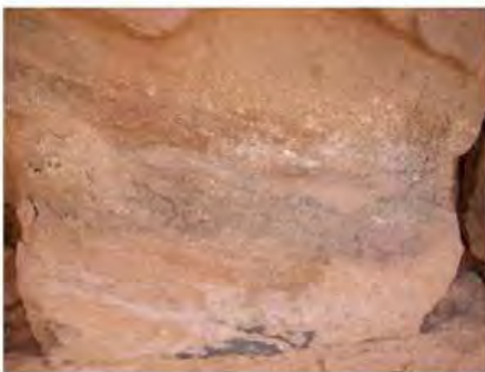
DSCN4005.JPG, The Kiosk - Naqaa, Naqaa, Degradation of Stone/ Masonry Elements, Inappropriate/Inexistent Site Drainage
