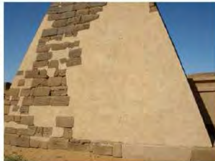
DSCN3828.JPG, Failure of Past Repair Work, Southern Cemetery
