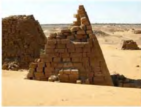
DSCN3852.JPG, Structural Deterioration of Pyramids, Southern Cemetery
