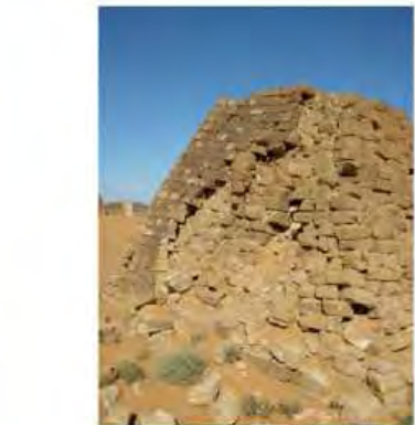
DSCN3863.JPG, Structural Deterioration of Pyramids, Southern Cemetery
