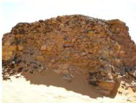
DSCN3739.JPG, Structural Deterioration of Pyramids, Northern Cemetery
