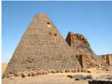
DSCN3808.JPG, Structural Deterioration of Pyramids, Southern Cemetery
