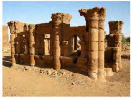
DSCN3998.JPG, The Kiosk - Naqaa, Naqaa, Degradation of Stone/ Masonry Elements, Inappropriate/Inexistent Site Drainage
