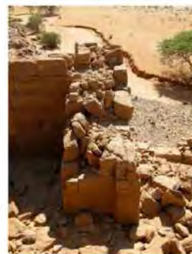
DSCN4154.JPG, Naqaa, Temple F, Structural Instability of Walls/Collapse of Archaeological Features, Structural Instability of Walls/Collapse of Archaeological Features
