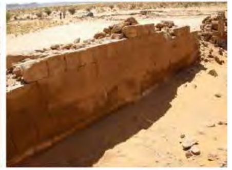
DSCN4175.JPG, Musawwarat - Great Enclosure, Restoration Works, Degradation of Stone/Masonry Elements, Salt Crystallization
