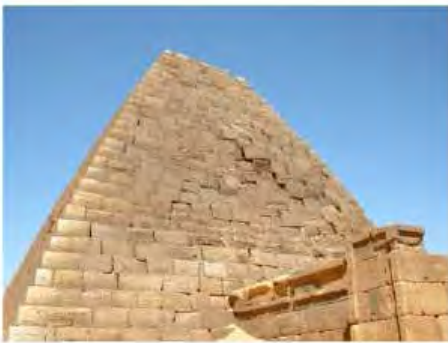
DSCN3765.JPG, Structural Deterioration of Pyramids, Northern Cemetery
