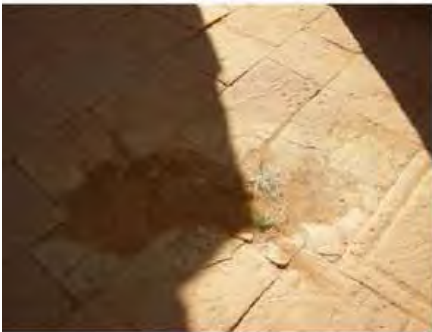
DSCN4100.JPG, Naqaa, Amun Temple, Inappropriate/Inexistent Site Drainage, Vegetation Damage
