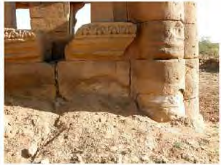
DSCN4001.JPG, The Kiosk - Naqaa, Naqaa, Degradation of Stone/ Masonry Elements, Inappropriate/Inexistent Site Drainage
