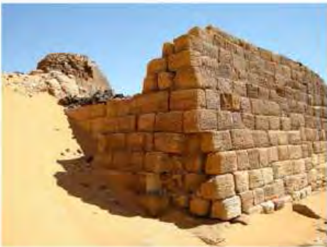
DSCN3753.JPG, Structural Deterioration of Pyramids, Northern Cemetery
