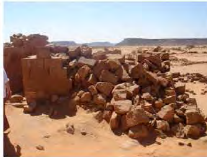
DSC06205.JPG, Musawwarat - Great Enclosure, Structural Instability of Walls/Collapse of Archaeological Features, Structural Instability of Walls/Collapse of Archaeological Features
