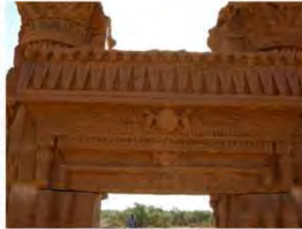
DSCN4006.JPG, The Kiosk - Naqaa, Naqaa, Structural Instability of Walls/Collapse of Archaeological Features
