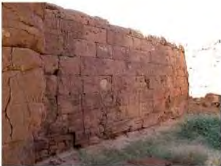
DSCN4024.JPG, Lion Temple B300 - Naqaa, Naqaa, Degradation of Stone/Masonry Elements, Inappropriate/Inexistent Site Drainage, Vegetation Damage
