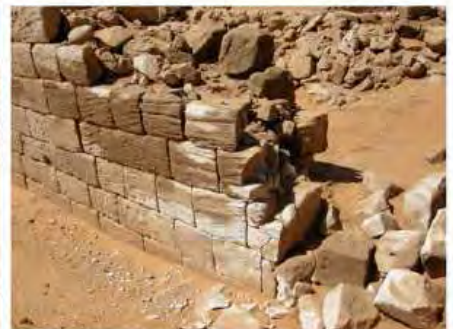
DSCN4172.JPG, Musawwarat - Great Enclosure, Degradation of Stone/Masonry Elements, Structural Instability of Walls/Collapse of Archaeological Features, Structural Instability of Walls/Collapse of Archaeological Features, Salt Crystallization
