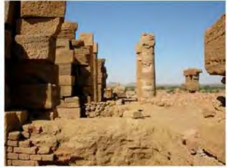
DSCN4111.JPG, Naqaa, Amun Temple, Deterioration of Ancient Mud Structures
