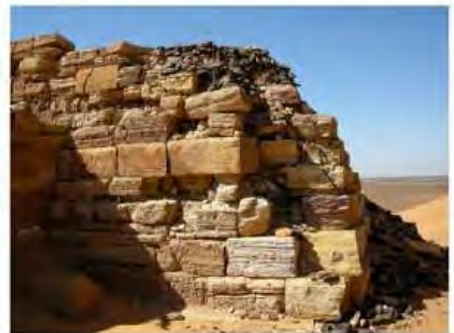
DSCN3728.JPG, Structural Deterioration of Pyramids, Northern Cemetery
