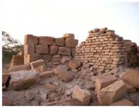
DSCN3978.JPG, Structural Instability of Walls/Collapse of Archaeological Features, Degradation of Stone/Masonry Elements, Inappropriate Dumping of Excavation Spoils, Inappropriate/Inexistent Site Drainage, Royal City
