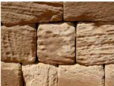
DSCN4170.JPG, Musawwarat - Great Enclosure, Degradation of Stone/Masonry Elements, Salt Crystallization
