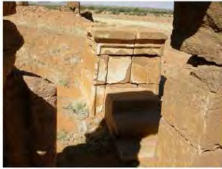
DSCN4123.JPG, Naqaa, Amun Temple, Exposure and Deterioration of Ancient Plasters, Inappropriate/Inexistent Site Drainage
