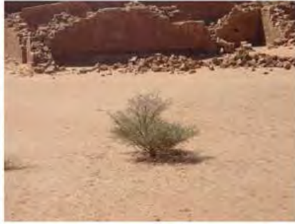
DSC06190.JPG, Musawwarat - Great Enclosure, Structural Instability of Walls/Collapse of Archaeological Features, Structural Instability of Walls/Collapse of Archaeological Features
