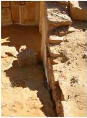
DSCN4120.JPG, Naqaa, Amun Temple, Exposure and Deterioration of Ancient Plasters, Inappropriate/Inexistent Site Drainage
