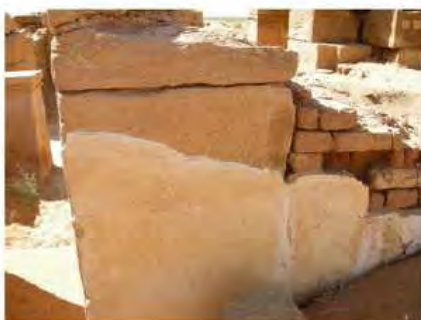
DSCN4117.JPG, Naqaa, Amun Temple, Exposure and Deterioration of Ancient Plasters, Deterioration of Ancient Mud Structures
