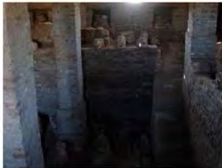
DSC06248.JPG, Inappropriate/Inexistent Site Drainage, Degradation of Stone/Masonry Elements, Royal City
