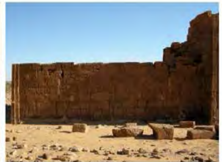
DSCN4030.JPG, Lion Temple B300 - Naqaa, Naqaa, Degradation of Stone/Masonry Elements, Inappropriate/Inexistent Site Drainage
