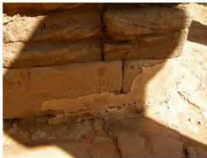
DSCN4098.JPG, Naqaa, Amun Temple, Exposure and Deterioration of Ancient Plasters, Degradation of Stone/Masonry Elements
