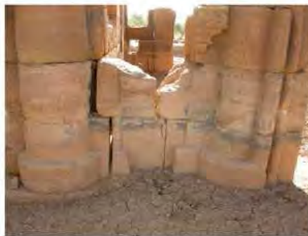
DSCN4007.JPG, The Kiosk - Naqaa, Naqaa, Degradation of Stone/ Masonry Elements, Inappropriate/Inexistent Site Drainage
