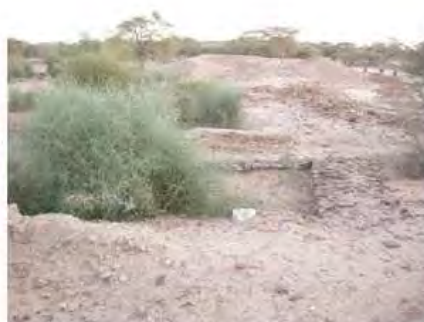
DSCN3951.JPG, Vegetation Damage, Inappropriate/Inexistent Site Drainage, Inappropriate Dumping of Excavation Spoils, Royal City
