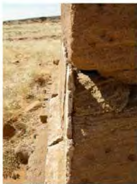
DSCN4081.JPG, Naqaa, Amun Temple, Exposure and Deterioration of Ancient Plasters
