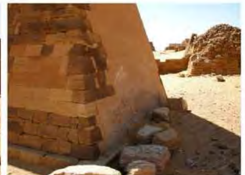
DSCN3779.JPG, Failure of Past Repair Work, Henkel Restoration, Salt Crystallization, Northern Cemetery
