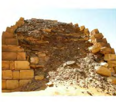
DSCN3742.JPG, Structural Deterioration of Pyramids, Northern Cemetery
