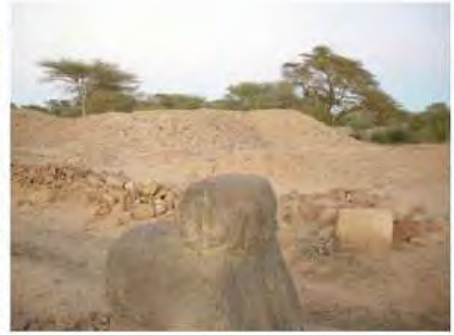
DSCN3955.JPG, Inappropriate Dumping of Excavation Spoils, Inappropriate/Inexistent Site Drainage, Royal City
