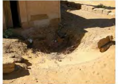
DSCN3835.JPG, Water Damage, Southern Cemetery
