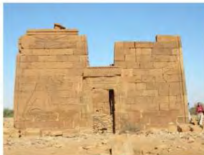
DSCN4012.JPG, Naqaa, Inappropriate/Inexistent Site Drainage
