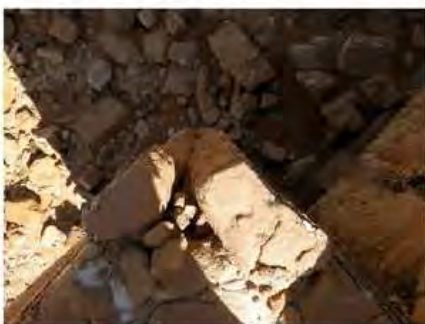
DSCN4157.JPG, Naqaa, Temple F, Structural Instability of Walls/Collapse of Archaeological Features, Structural Instability of Walls/Collapse of Archaeological Features
