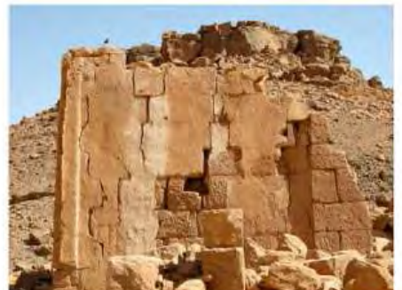
DSCN4142.JPG, Naqaa, Temple F, Structural Instability of Walls/Collapse of Archaeological Features, Structural Instability of Walls/Collapse of Archaeological Features, Exposure and Deterioration of Ancient Plasters
