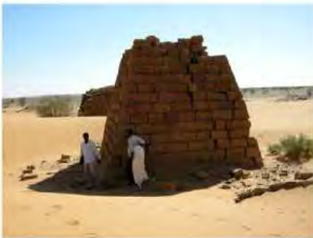
DSCN3860.JPG, Structural Deterioration of Pyramids, Southern Cemetery
