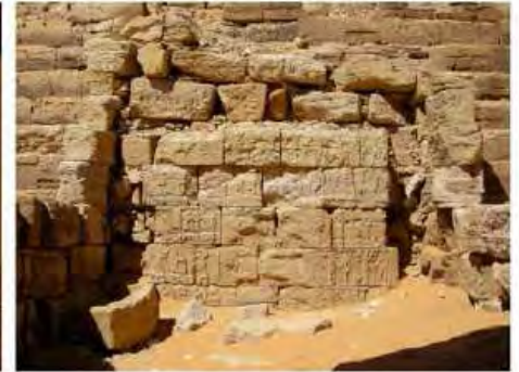
DSCN3773.JPG, Exposure and Deterioration of Ancient Reliefs, Northern Cemetery
