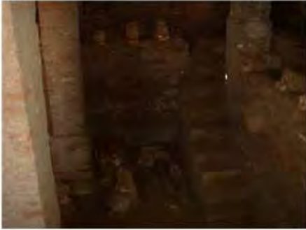
DSC06258.JPG, Inappropriate/Inexistent Site Drainage, Royal City
