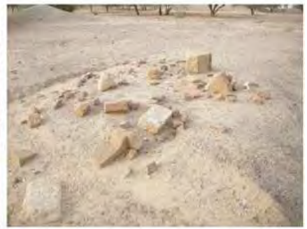
DSCN3943.JPG, Degradation of Stone/Masonry Elements, Royal City
