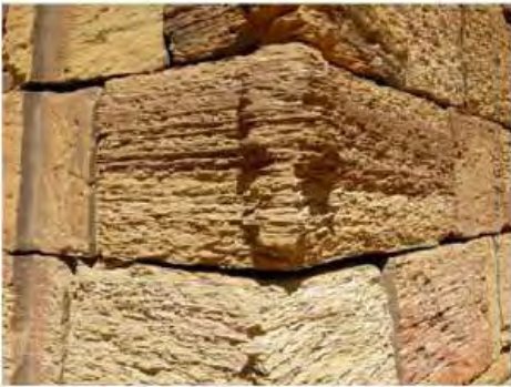
DSCN3750.JPG, Degradation of Stone/Masonry Elements, Northern Cemetery
