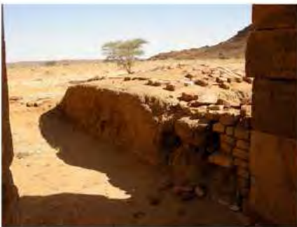
DSCN4102.JPG, Naqaa, Amun Temple, Deterioration of Ancient Mud Structures
