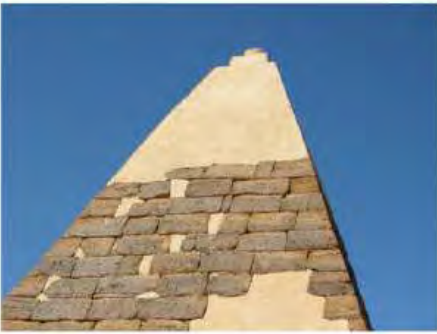
DSCN3830.JPG, Failure of Past Repair Work, Southern Cemetery
