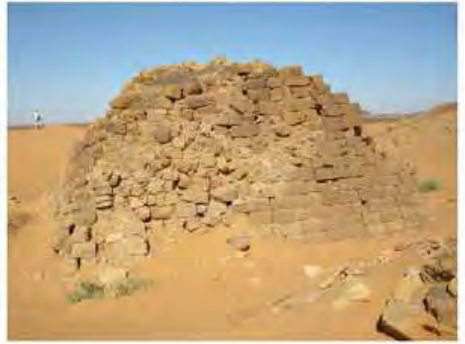
DSCN3847.JPG, Structural Deterioration of Pyramids, Southern Cemetery
