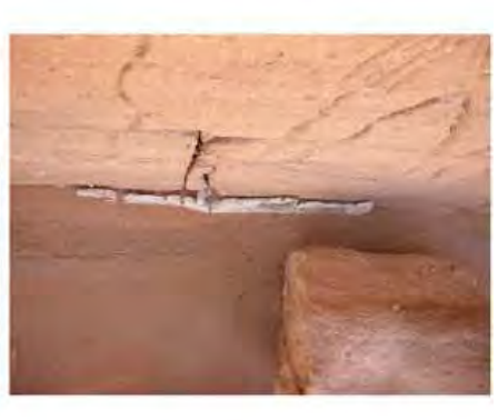
DSCN4085.JPG, Naqaa, Amun Temple, Exposure and Deterioration of Ancient Plasters
