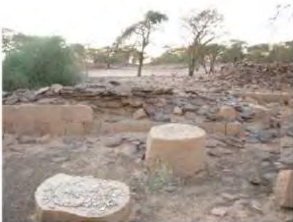
DSCN3947.JPG, Structural Instability of Walls/Collapse of Archaeological Features, Degradation of Stone/Masonry Elements, Royal City
