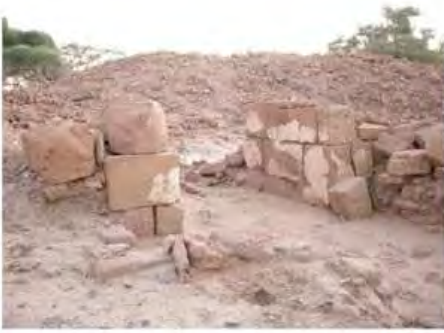
DSCN3965.JPG, Inappropriate Dumping of Excavation Spoils, Exposure and Deterioration of Ancient Plasters, Degradation of Stone/Masonry Elements, Structural Instability of Walls/Collapse of Archaeological Features, Royal City
