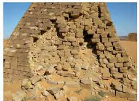
DSCN3886.JPG, Structural Deterioration of Pyramids, Southern Cemetery
