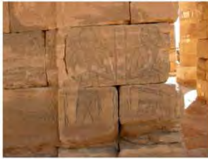
DSCN4096.JPG, Naqaa, Amun Temple, Degradation of Stone/Masonry Elements, Structural Instability of Walls/Collapse of Archaeological Features
