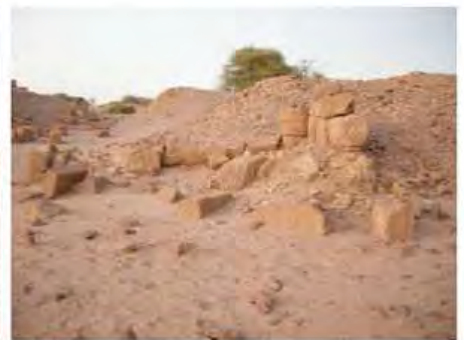
DSCN3976.JPG, Degradation of Stone/Masonry Elements, Structural Instability of Walls/Collapse of Archaeological Features, Inappropriate Dumping of Excavation Spoils, Inappropriate/Inexistent Site Drainage, Royal City
