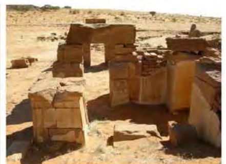
DSCN4119.JPG, Naqaa, Amun Temple, Exposure and Deterioration of Ancient Plasters, Inappropriate/Inexistent Site Drainage
