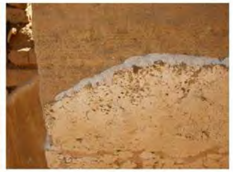
DSCN4114.JPG, Naqaa, Amun Temple, Exposure and Deterioration of Ancient Plasters
