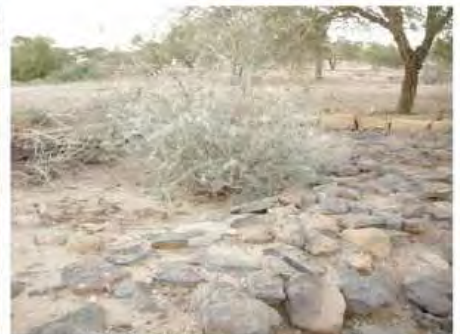
DSCN3940.JPG, Vegetation Damage, Structural Instability of Walls/Collapse of Archaeological Features, Royal City
