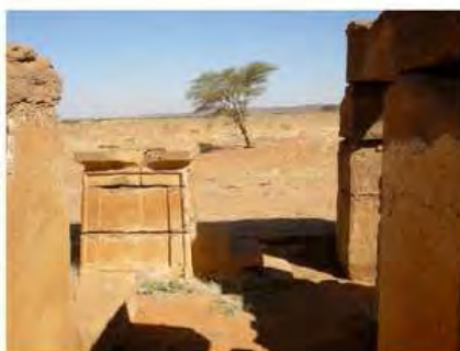
DSCN4112.JPG, Naqaa, Amun Temple, Exposure and Deterioration of Ancient Plasters, Inappropriate/Inexistent Site Drainage
