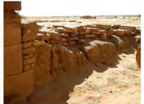
DSCN4101.JPG, Naqaa, Amun Temple, Structural Instability of Walls/Collapse of Archaeological Features, Degradation of Stone/ Masonry Elements
