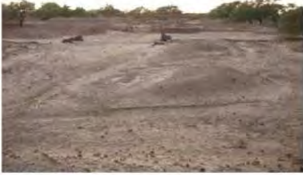
DSCN3953.JPG, Inappropriate/Inexistent Site Drainage, Inappropriate Dumping of Excavation Spoils, Royal City
