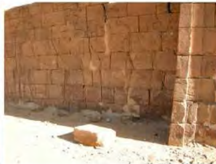
DSCN4029.JPG, Lion Temple B300 - Naqaa, Naqaa, Degradation of Stone/Masonry Elements, Inappropriate/Inexistent Site Drainage
