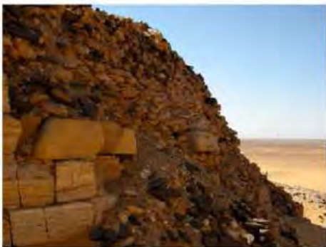
DSCN3738.JPG, Structural Deterioration of Pyramids, Northern Cemetery
