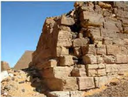
DSCN3711.JPG, Structural Deterioration of Pyramids, Northern Cemetery
