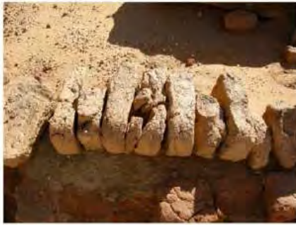
DSCN4090.JPG, Naqaa, Amun Temple, Degradation of Stone/Masonry Elements, Structural Instability of Walls/Collapse of Archaeological Features
