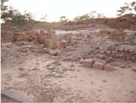
DSCN3968.JPG, Structural Instability of Walls/Collapse of Archaeological Features, Inappropriate Dumping of Excavation Spoils, Inappropriate/Inexistent Site Drainage, Royal City
