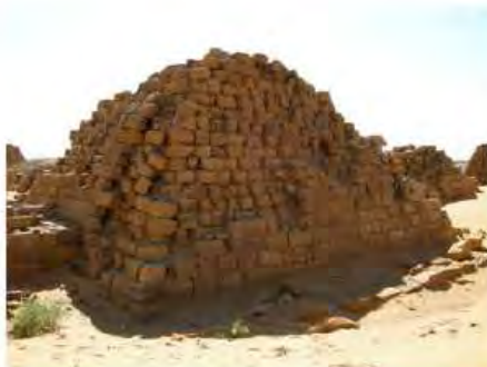
DSCN3840.JPG, Structural Deterioration of Pyramids, Southern Cemetery
