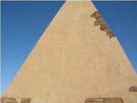
DSCN3833.JPG, Failure of Past Repair Work, Southern Cemetery
