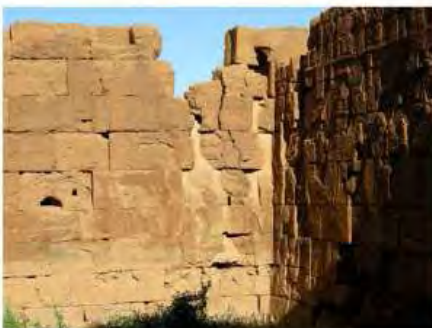
DSCN4028.JPG, Lion Temple B300 - Naqaa, Naqaa, Inappropriate/Inexistent Site Drainage, Vegetation Damage
