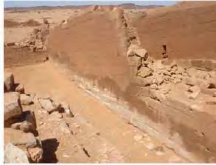
DSC06202.JPG, Musawwarat - Great Enclosure, Degradation of Stone/Masonry Elements, Salt Crystallization
