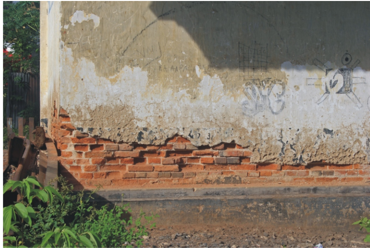
Image.4.11 Cement deterioration due to climatic tropical condition at Batu Tabal Train Station
