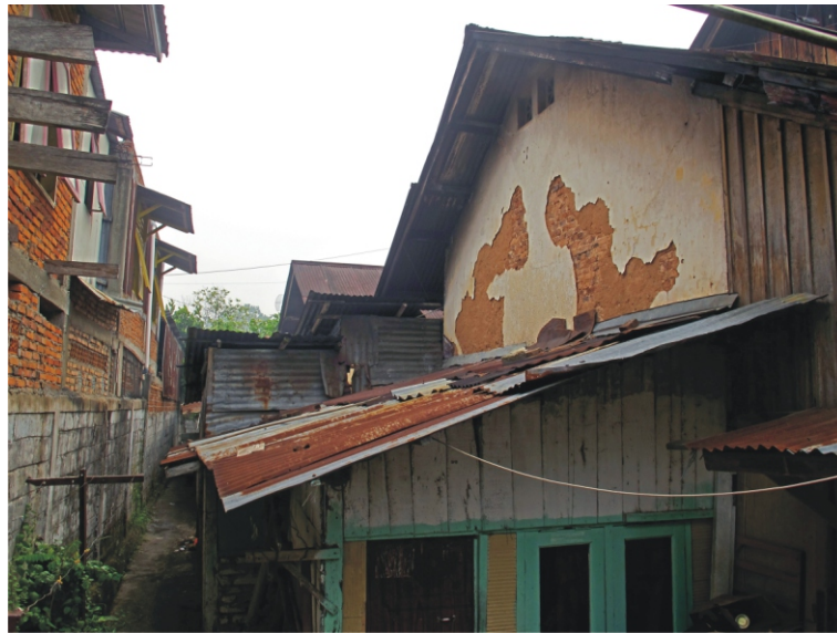
Image.4.5 Unsuitable renovation works in Tangsi Baru area of new room addition
