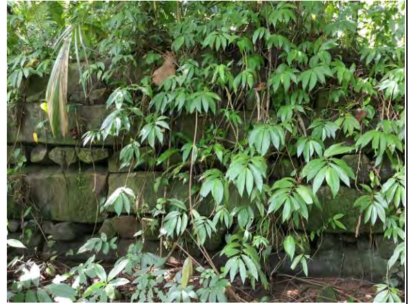
Fig.8: Large amount of biological growth on structures
