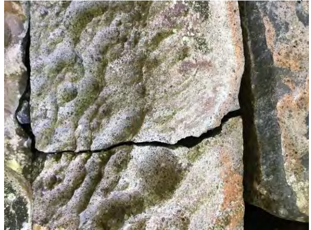
Fig 14: Cracked stone with no need to prop
