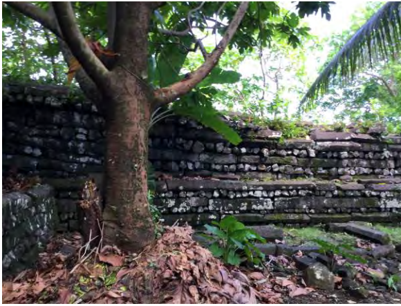
Fig.7: Large tree close to wall structure
