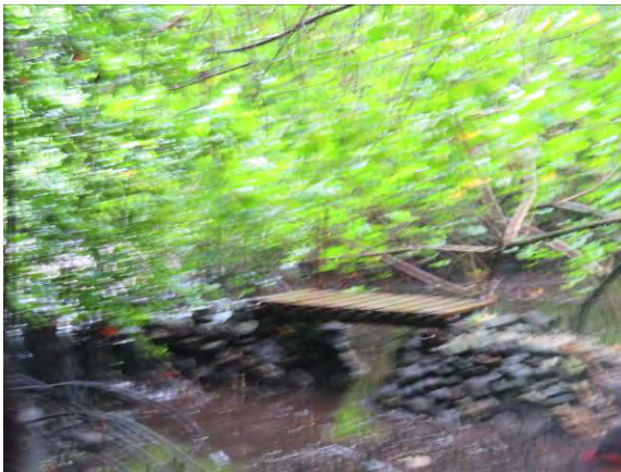
Fig 17: One of the bridges causing a restriction to water movement
