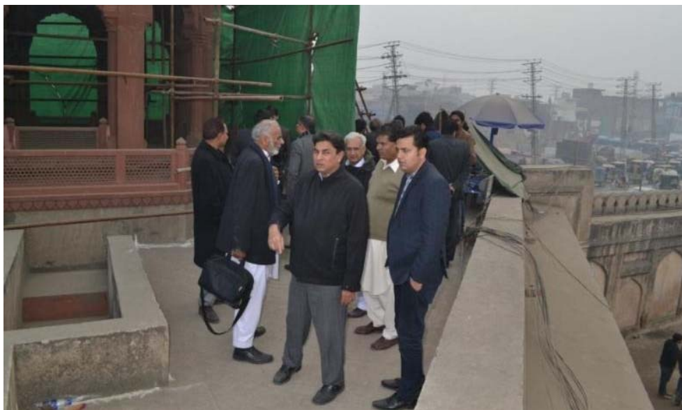
Visit of Advisory Committee at Shalamar Gardens to ensure the Safety Measures during construction of Orange Line Metro Train Track
