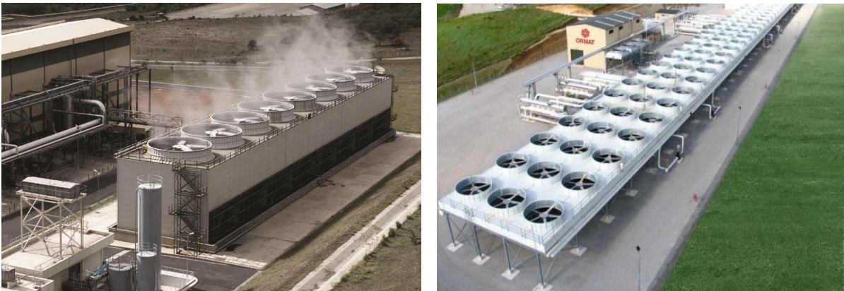
Figure 3-1: Turbine Hall and Evaporative Cooling Tower (left). Air cooling for 20MW plant (right)
