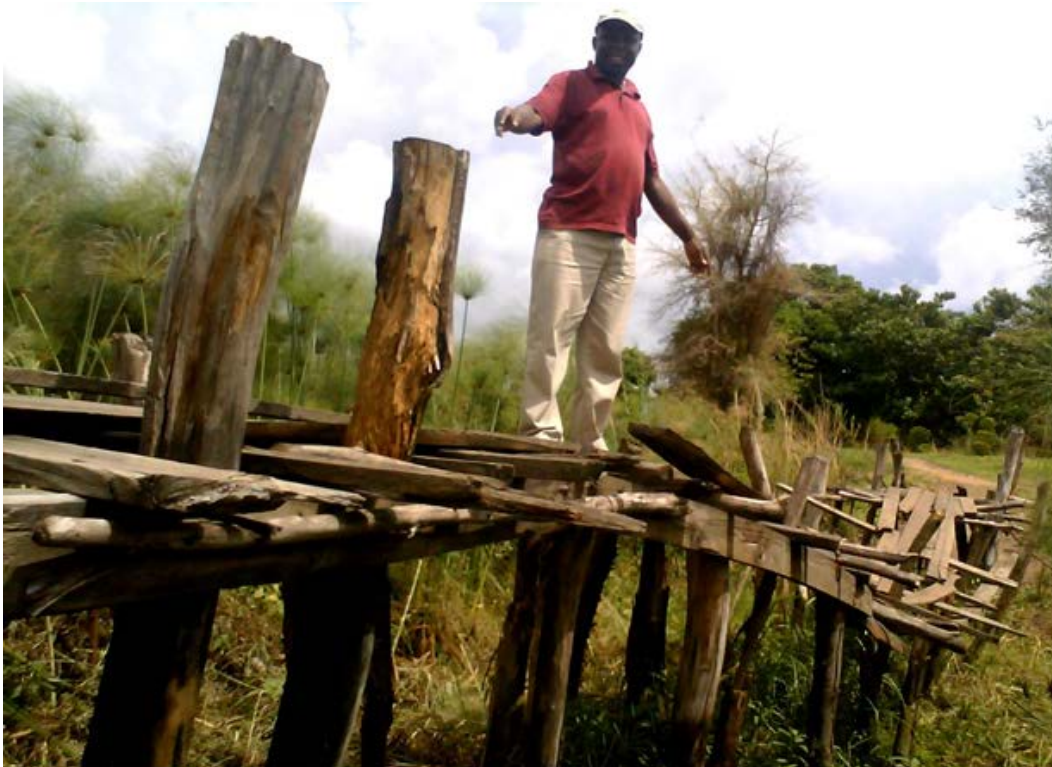
A footpath Kacherenje bridge in Salima TA Maganga, GVH Mgawi before maintenance
