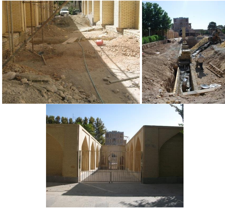
Figure 14. The Royal road in restoration phase (left and middle)- completed project (right)
