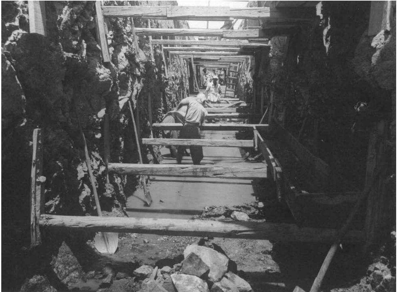
Figs 1.29 - 1.30: Eritrean labourers digging storm water drainage and preparing earthworks in the suburb of Gbeza Banda.
