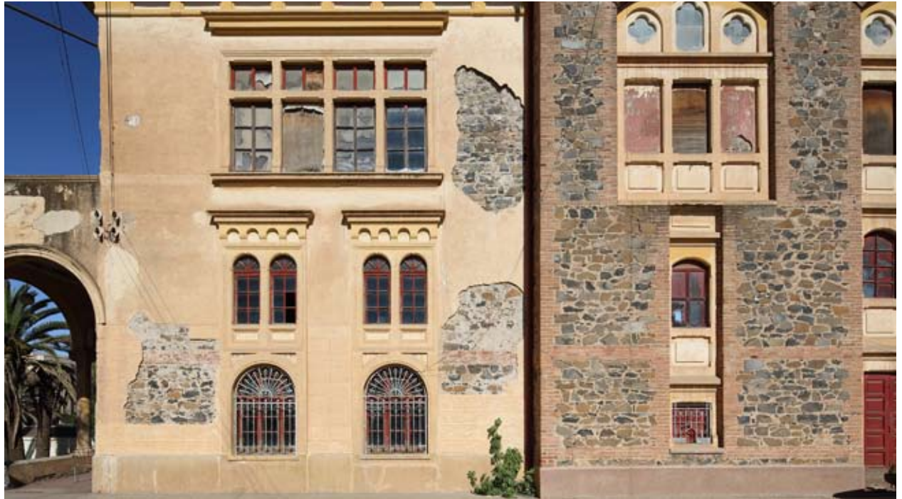
Fig 1.4: The side elevation of Teatro Asmara revealing the different types of basalt blocks used in construction. Dressed blocks are used on exposed surfaces combined with brick and reinforced concrete members around openings, while rough blocks are used on plastered walls. A raised band of plaster at the base of the building conceals the larger basalt blocks used in the foundations and to prevent rising damp.
