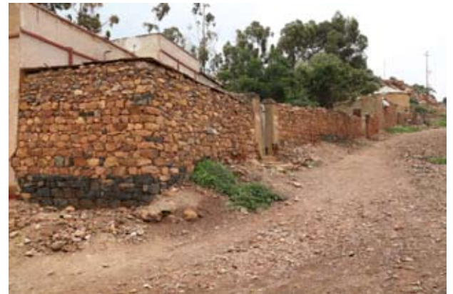
Figs 1.23 - 1.25: (below) Examples in Asmara of the traditional building techniques used in three different domestic contexts that exploit the properties of basalt for foundations with lighter, softer, cheaper stone, such as sandstone, above.
