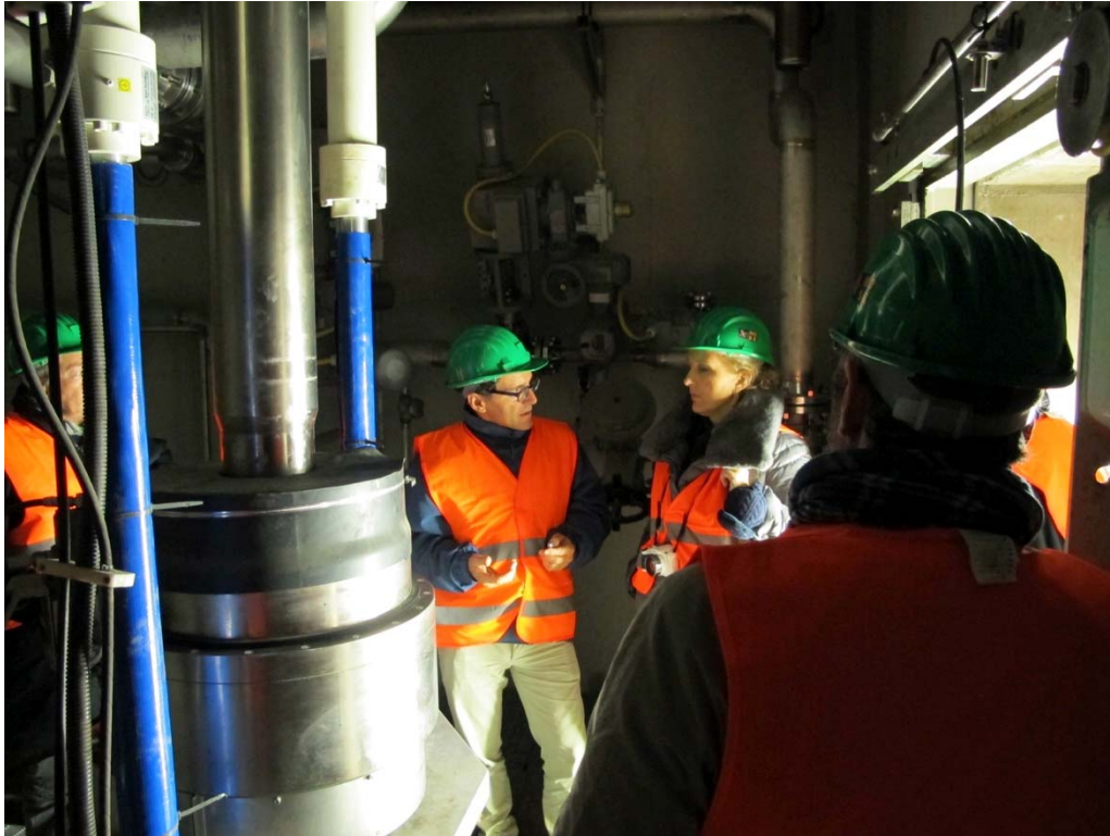
UNESCO mission at the hydraulic pumps of the MoSE system underneath the Lido Lagoon inlet. (Tobias Salathé, October 2015)
