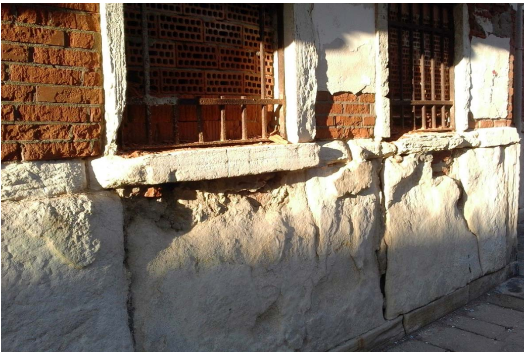
Palazzo Minotto, Fondamenta Briati (Orsoduro 2365-2371A): property of the Comune, closed and with bricked windows, abandoned and out of use since years, with important defects due to humidity (exterior and interior). (Bernhard Furrer, October 2015)
