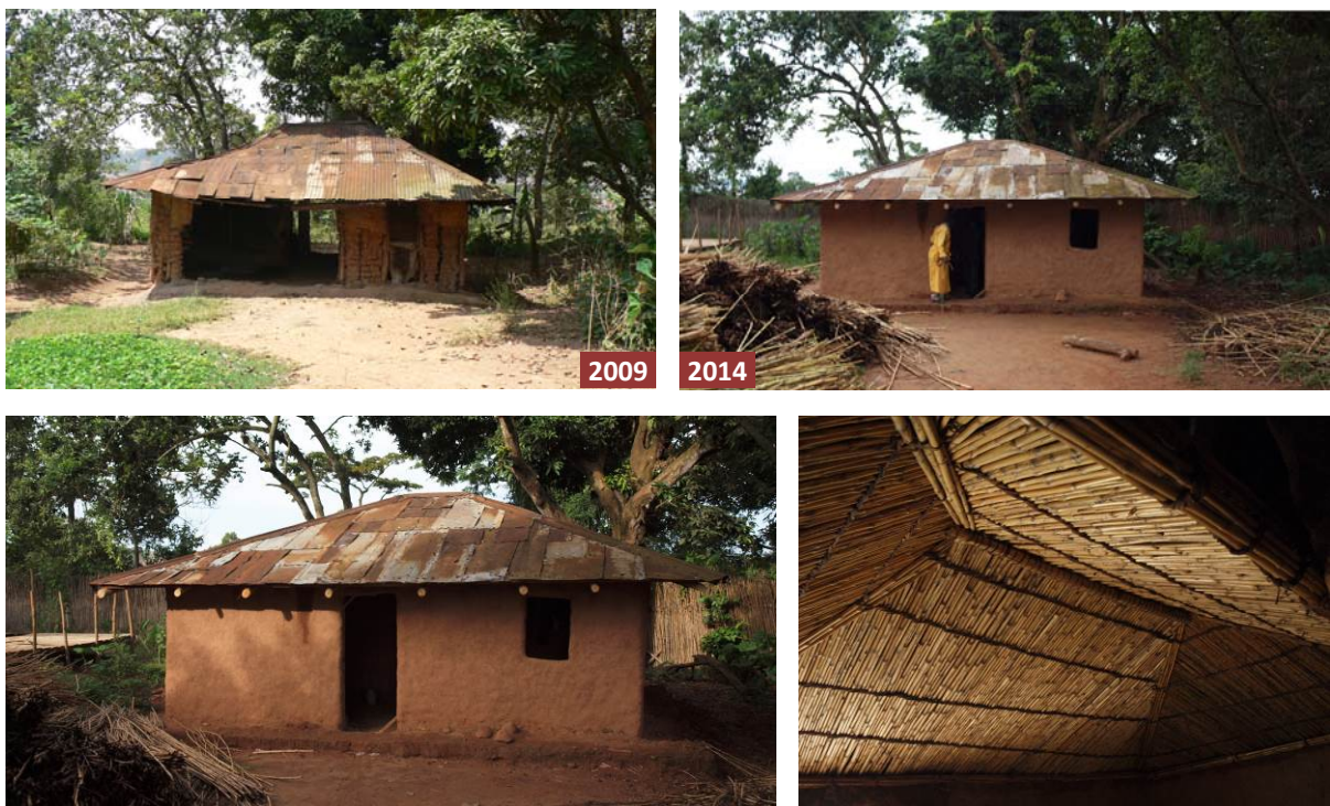
Wattle and daub house under restoration during the mission. This work is perfectly in line with the conservation and development of traditional skills
