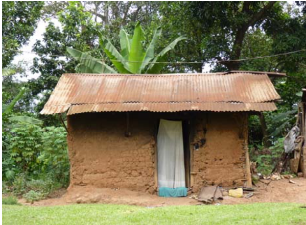
Mud house destroyed
