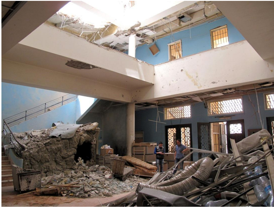
Destruction of the ceiling at the main entrance hall and damage to Paleolithic exhibit of finds from Jurf al-Ajla in the museum of Palmyra
