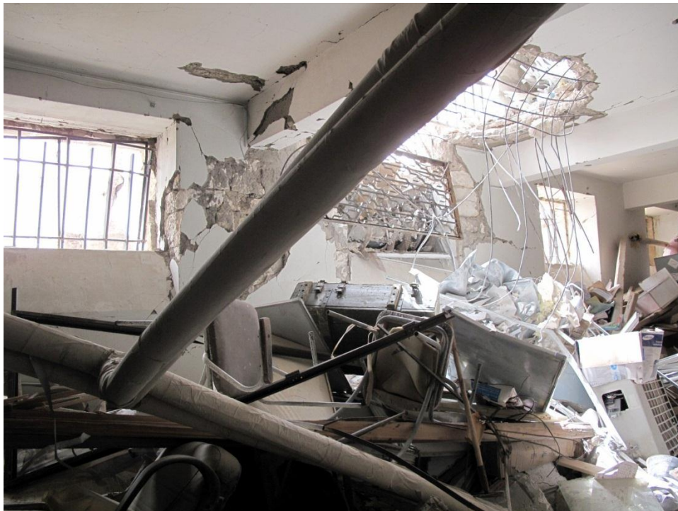
Destruction of the ceiling at the office room (2) in the museum of Palmyra
