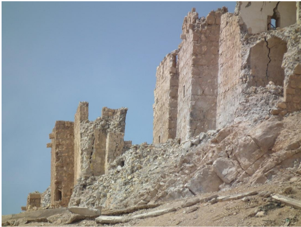
Close footage showing the collapsed of the southeastern curtain wall of Castle of Fakhral-Din al-Ma'ani
