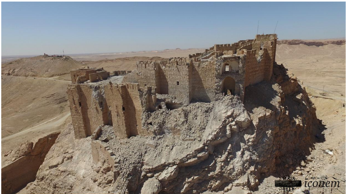
The southeastern curtain wall and the entrance of Castle of Fakhr-al-Din al-Ma'ani has suffered a major collapse
