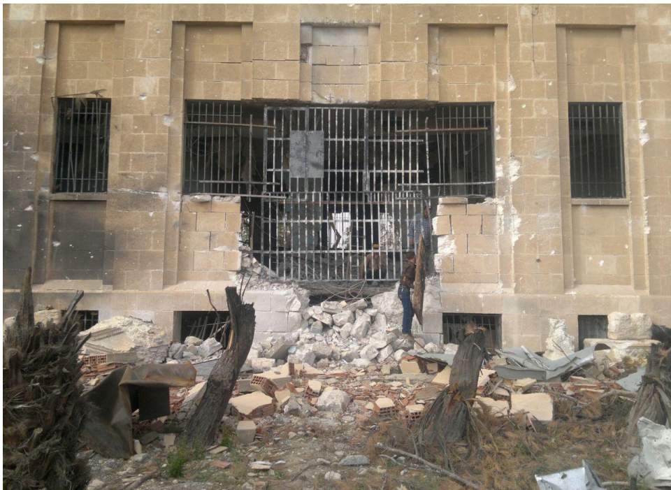
Slight damage to the background facade in the museum of Palmyra
