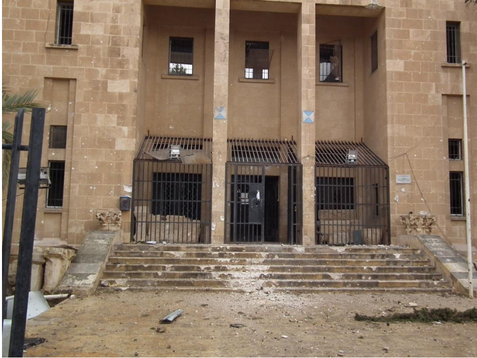
Slight damage to stairs and the walls of the main facade in the museum of Palmyra
