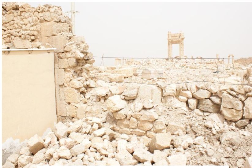
Section of outer modern western wall has partially collapsed.
