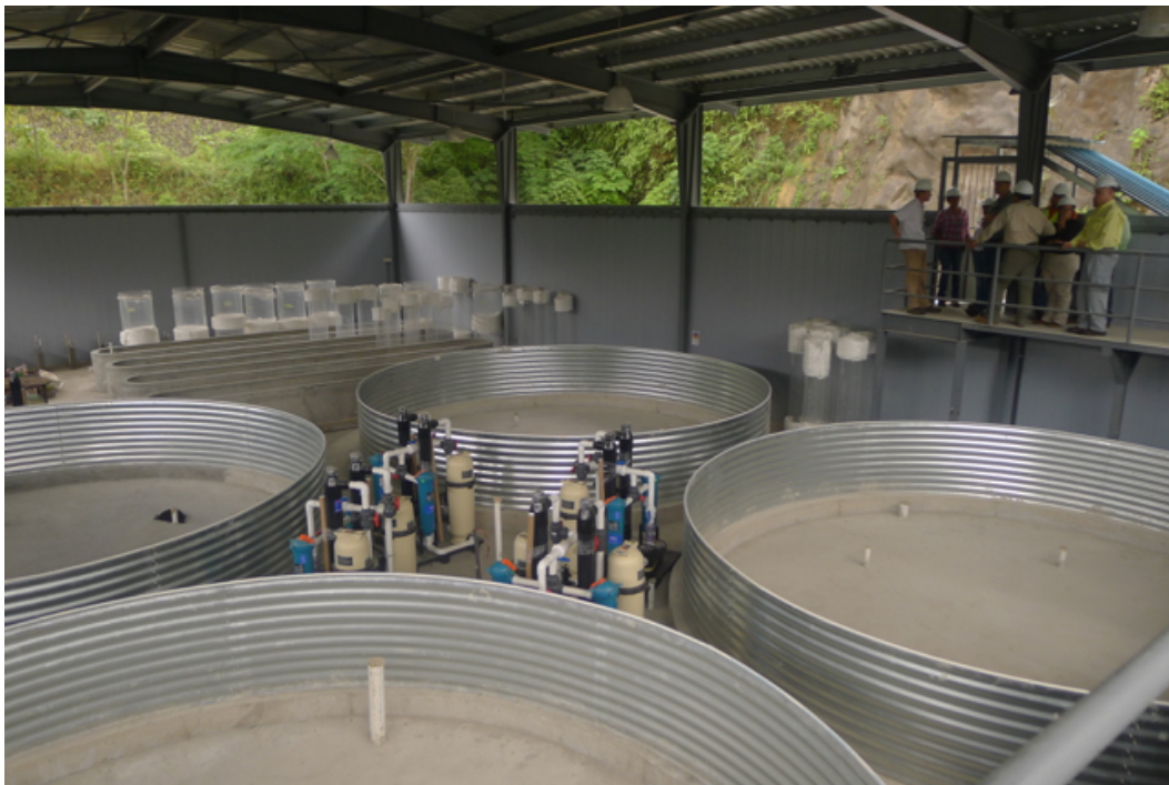
Hydrobiological station (for farming native fish) under construction near CHAN75 dam, 14 January (© Robert Hofstede).
